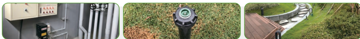
The Company installed a rainwater recycling pool on 11F of the Yanping building for watering plants on the roof.
