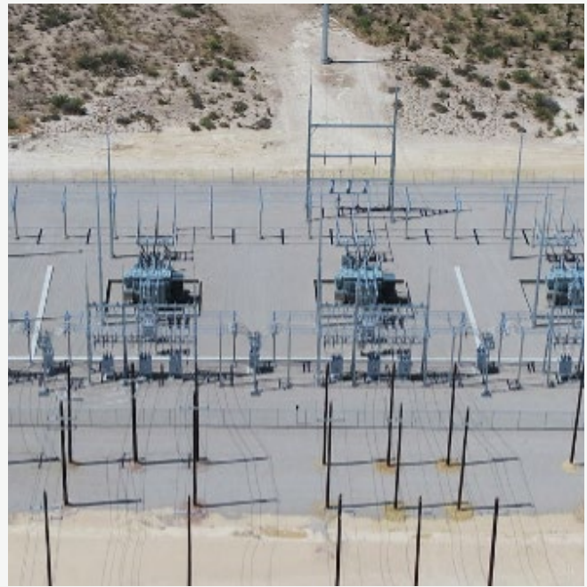
Substation: part of Coterra's electric infrastructure
