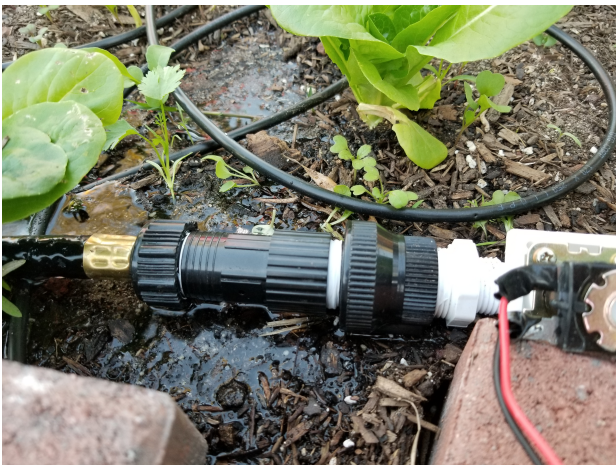
Fig. 7. Leaky hose connector with ill-fitting thread
