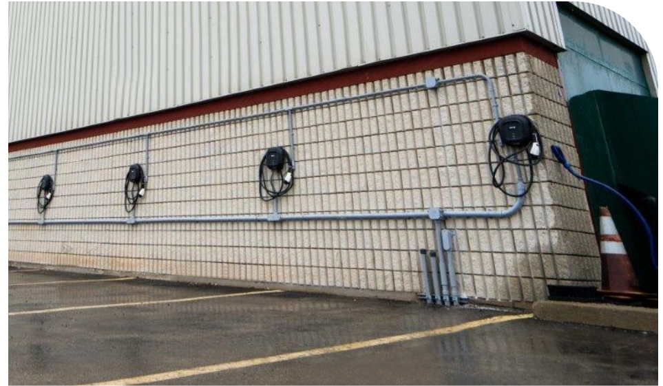
Charging infrastructure installed at our Burlington, Ontario, location in fall 2022
