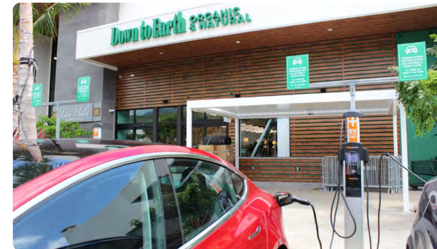
EV CHARGING STATIONS AT LAU HALA SHOPS (KAILUA, O'AHU)
