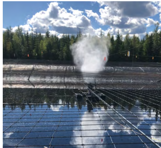
Leachate mister operating at the Silverberry Landfill.
