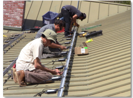
Residential Solar Installation, photo courtesy of SYCEO
