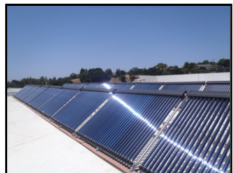
Solar thermal collectors at the Chumash Casino
