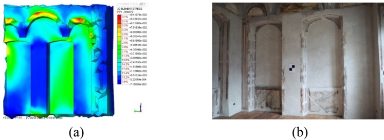
Figure 7: Tensile stresses in the dovecote tower wall (a) and cracks (b).
