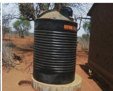
Plate 2: Plastic water tank
