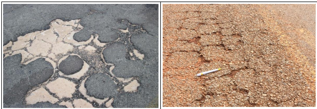
Figure A.6 Examples of Cemented Base Layers in an EG4 Stage of Deterioration
