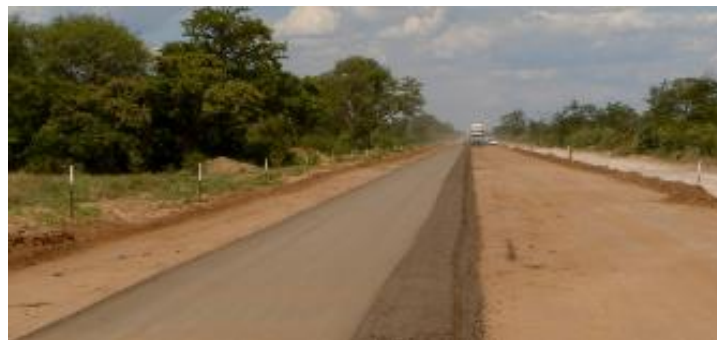
Figure 6.9 Uncompacted Strip of Material on the Centre-Line
