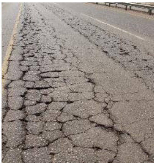
Figure 3.3 Severely Distressed Asphalt
