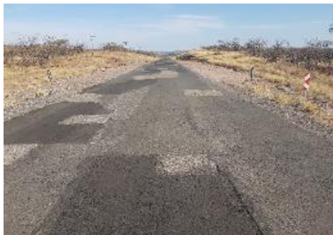
Figure 3.1 Extensively Patched Road
