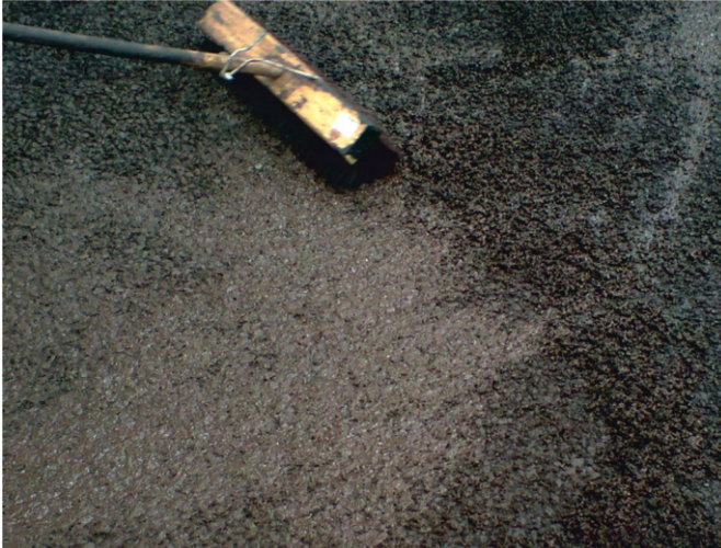
Photograph 37: Segregation (too coarse grading for texture treatment)
