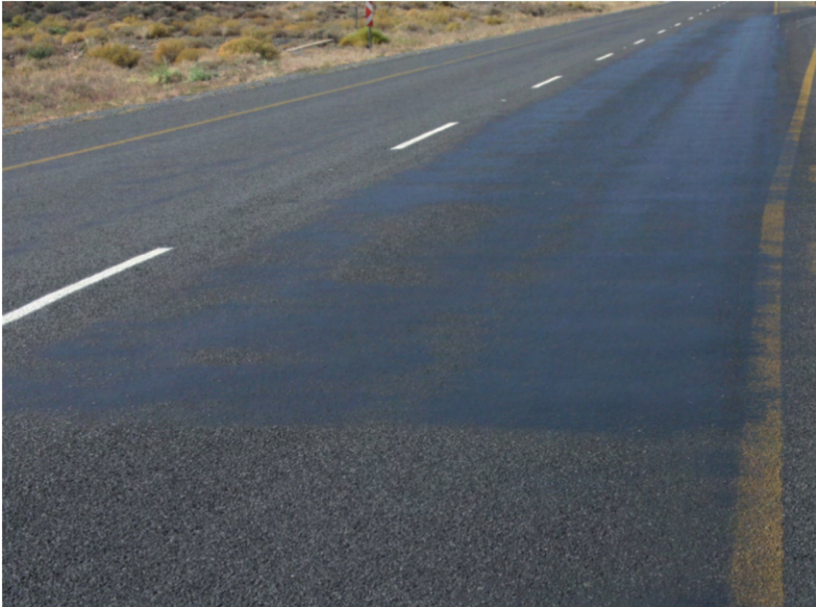
Photograph 40: Poor quality control on batch of Cape Seal slurry
