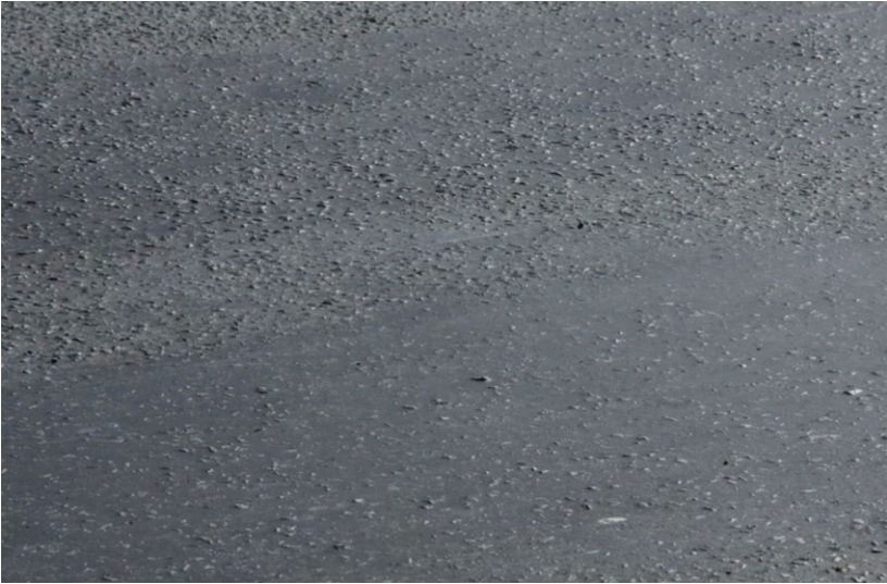
Photograph 39: Too high binder content
