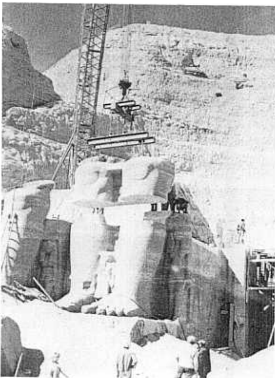
g. 23. - Pharaoh's knees being lifted after being cut loose. The lifting equipment is arranged so as to distribute the load of the block evenly on the four lifting-bars inserted (Cf. also Figure 25).
