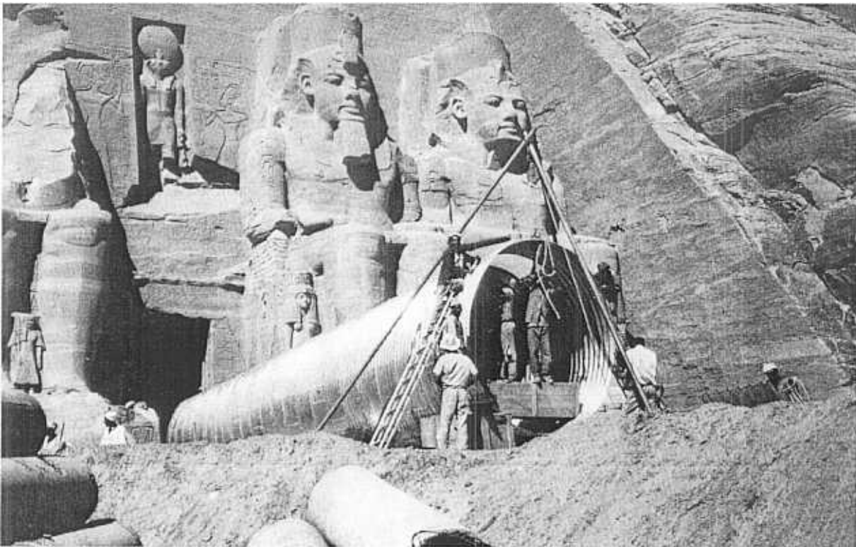
fig. 16. - In November, 1964, a steel culvert through the sandfill in front of the Great Temple was erected, to form an access to the temple rooms. The culvert access was in use until the beginning of 1966.
