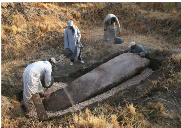
Interim measures: Reburying the block in gravel and sand to promote drainage.
