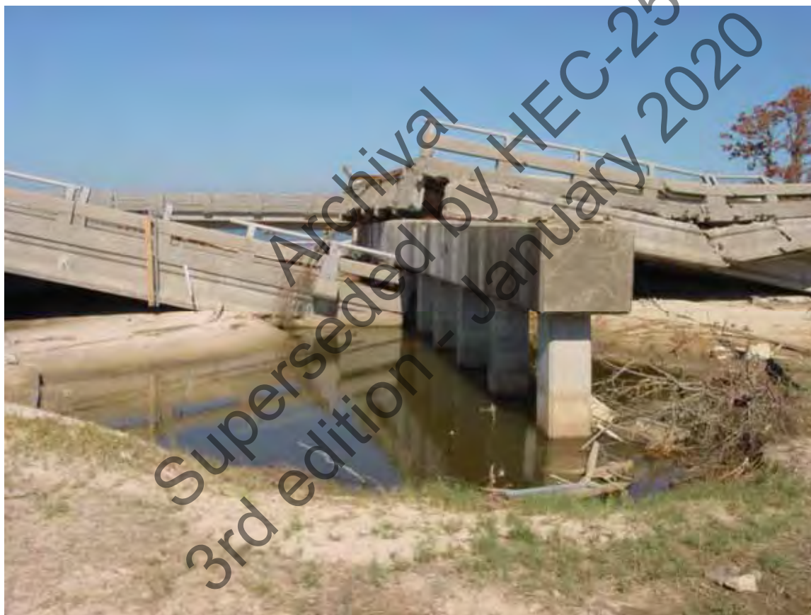
Figure 9.7. Wave scour hole formed by Hurricane Katrina.
