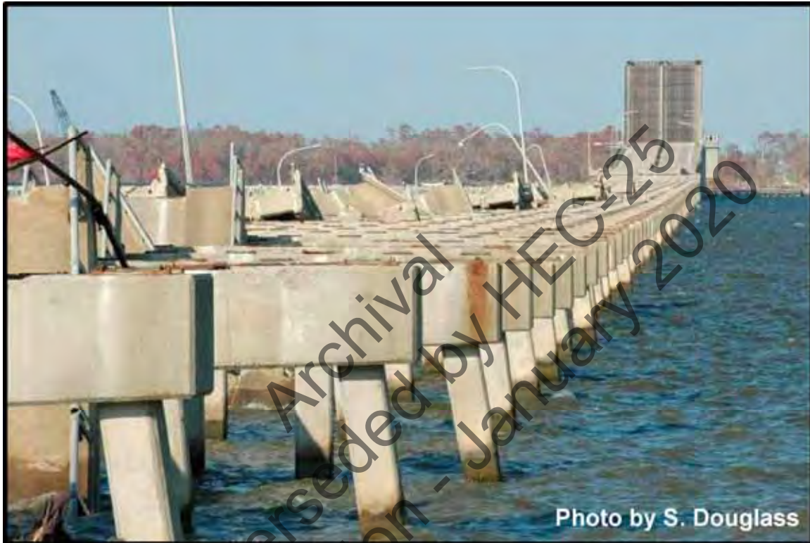
Figure 2.5. US Highway 90 bridge across Biloxi Bay, Mississippi, after Hurricane Katrina. (photo looking northeast from Biloxi 9/21/05).
