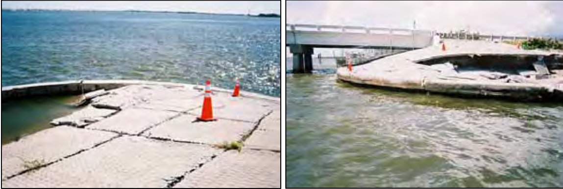
Figure 6.20. Example of rigid revetment failure on a coastal highway bridge approach
