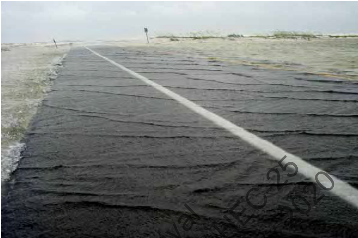
Figure 8.7. Weir-flow damage beginning. (Florida 399, Fort Pickens Road, Gulf Islands National Seashore; July 2005; FHWA photo).
