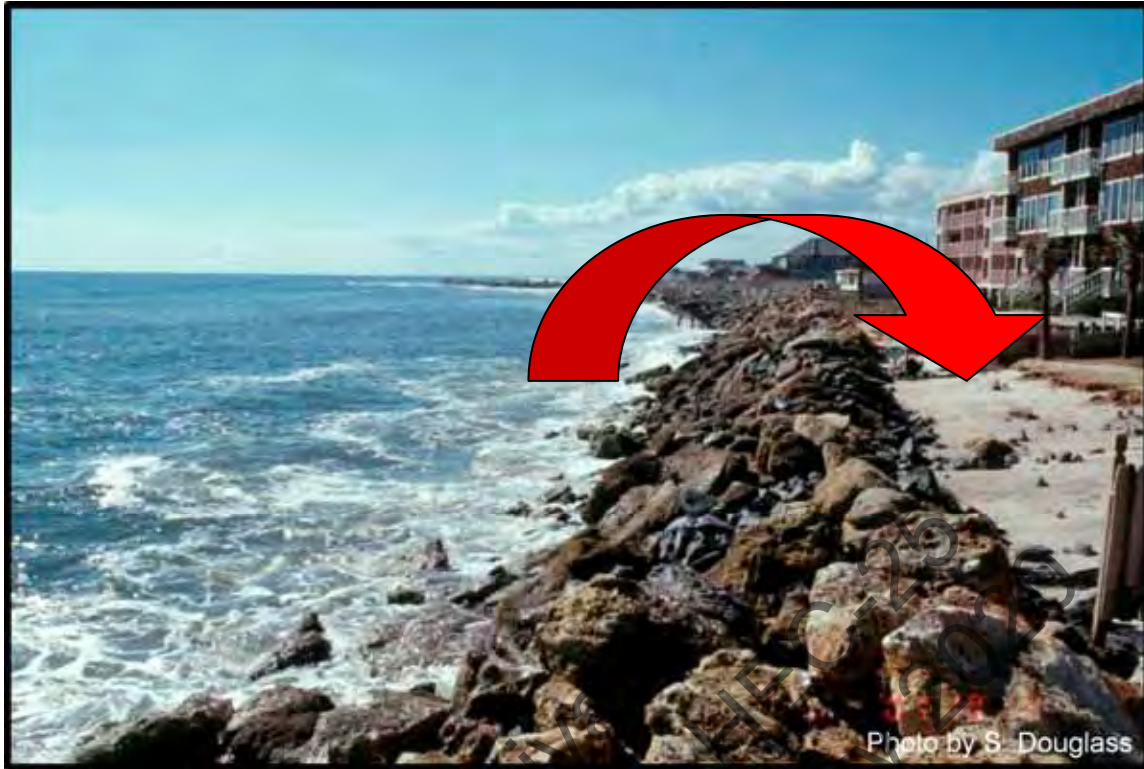
Figure 6.16. An example of splash damage behind seawall
