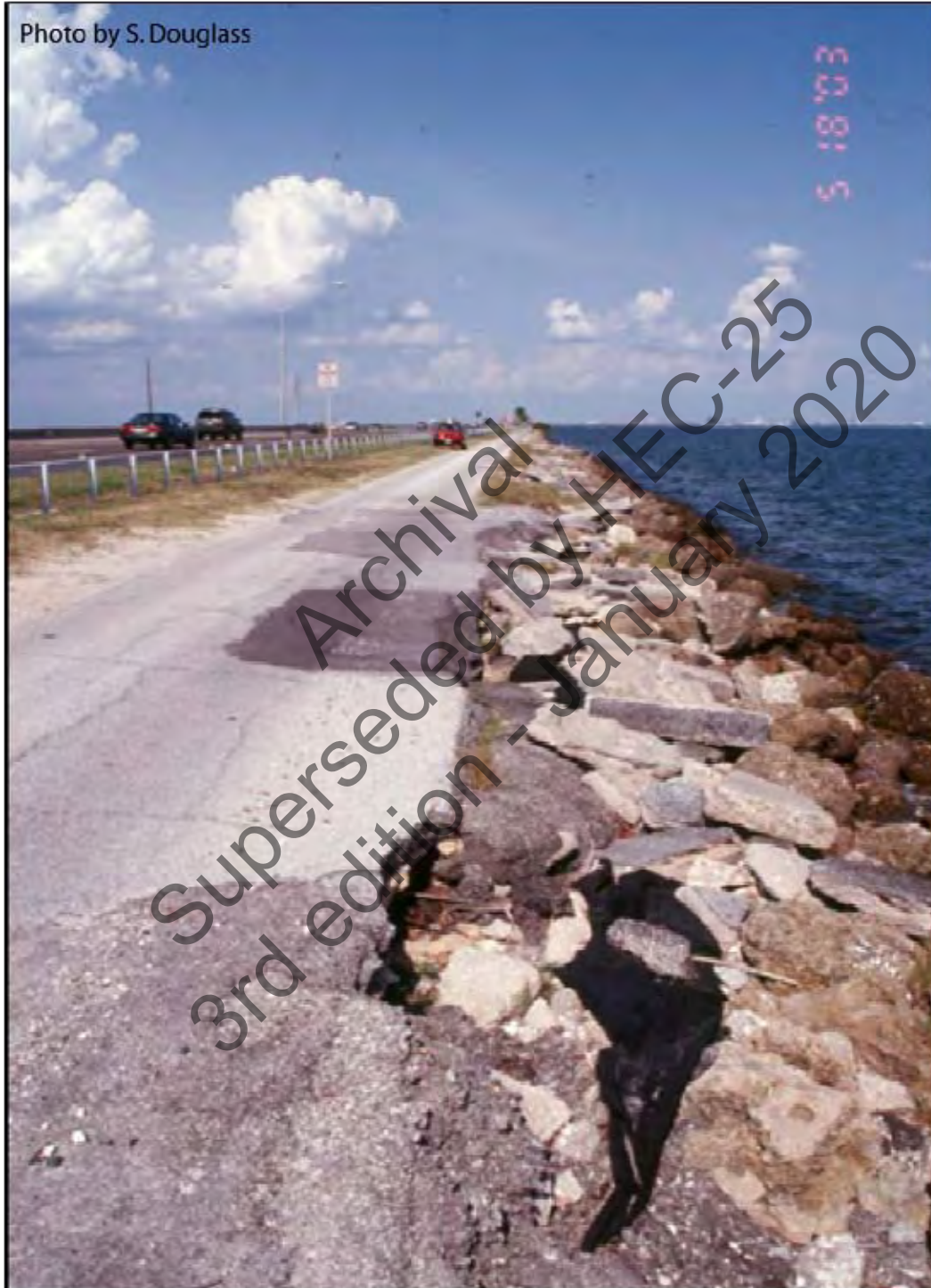
Figure 6.9. Revetment protecting a highway along a bay shoreline. Florida Highway 60, Tampa Bay, Florida (2003)
