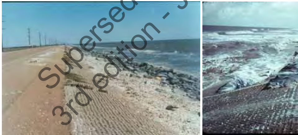
Figure 6.19. Example of failed block revetment (Louisiana Highway 87, circa 1980, USACE archives photos)
