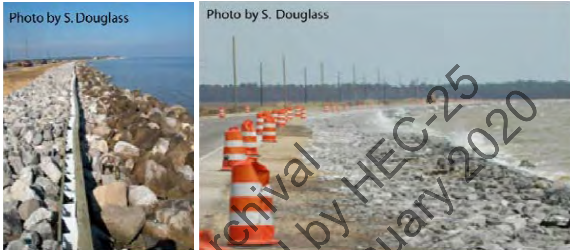
Figure 6.15. A revetment with rocks too small to withstand wave attack
