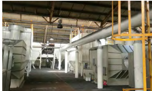
▲ Exhaust Gas Disposal Equipment
