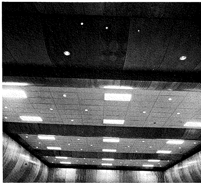
Fig. 9—Studio A ceiling at minimum height.
