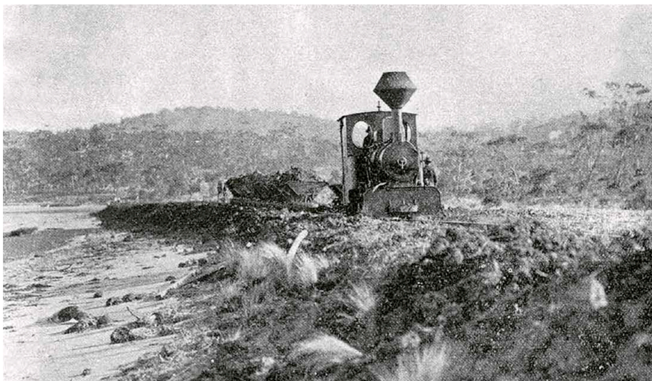
Tipping to spoil, Norfolk Bay, viewed from the land side' was the photographer's caption. After being excavated, dry material was removed by rail to both ends of the canal cut and dumped along the shoreline. This picture shows operations at the western end as seen by The Tasmanian Mail's special photographer. It is thought this scene is to the south of the existing canal swing bridge, on the shores of Dunalley Bay (part of Norfolk Bay). Tasmanian Mail, 2 June 1902 State Library of Tasmania
