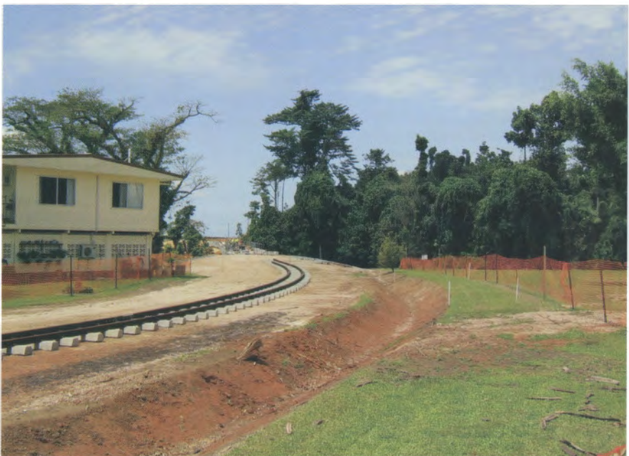
The line under construction from the new South Johnstone River bridge curves around close to some mill residences. 24 September 2008. Photo: Chris Hart
