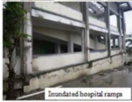
Inundated hospital ramps
