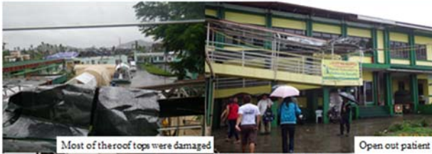
Most of the roof tops were damaged
