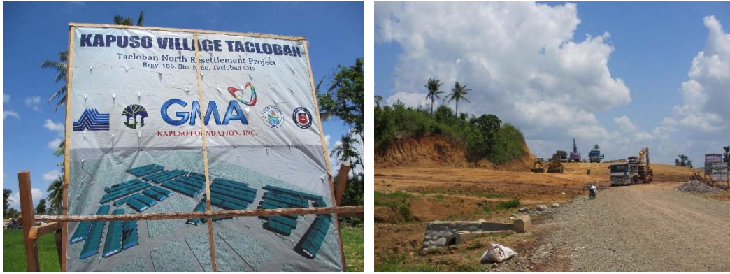
Fig. 11-10. Land development in March 2014 for the construction of permanent housing in the North Tacloban resettlement site.
