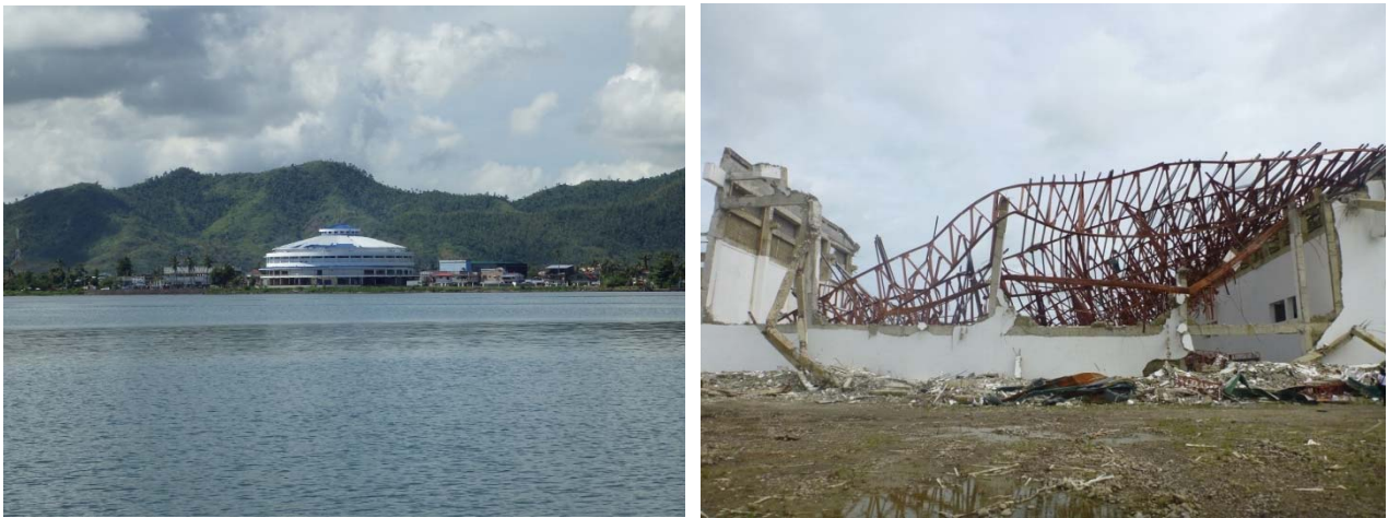
Fig. 2-11. Tacloban City Convention Center in Tacloban city (left) and Leyte Convention Center in Palo city (right).
