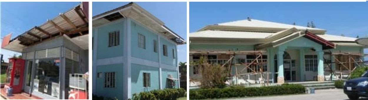
Fig. 9-12. Slightly damaged buildings (roof and windows) in Medellin, Cebu
