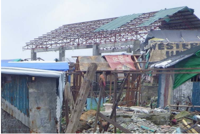
Fig.5-15. Roof damage at a public area in Tacloban.
