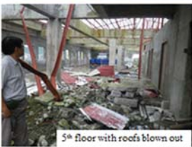
5th floor with roofs blown out
