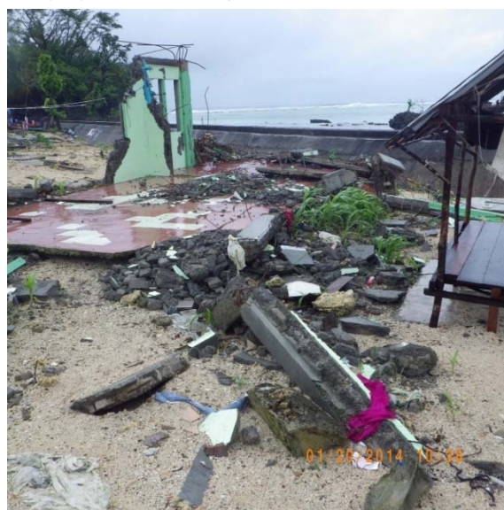
Fig.5-29. Debris from reinforced concrete house along coast in Hernani.
