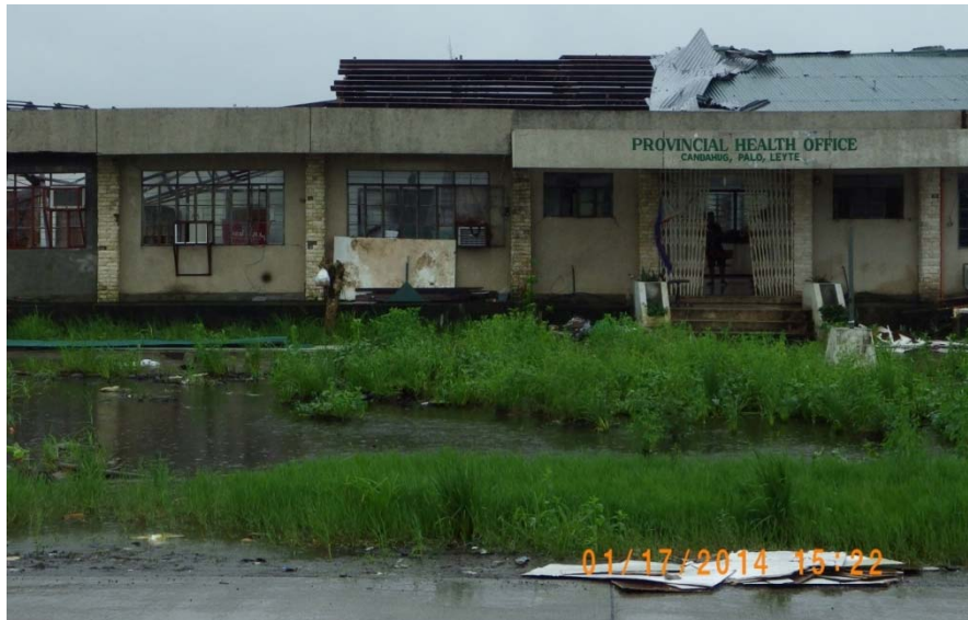
Fig.5-17. Roof damage at a hospital in Palo (south of Tacloban).
