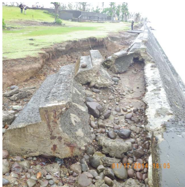
Fig.5-31. Seawall damage at the MacArthur Memorial south of Tacloban Airport. Crest height 3 m above Mean Sea Level.
