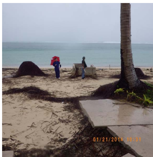
Fig.5-22. Damage near Guiuan PAGASA station. Damaged foundation located 4 m above Mean Sea Level.
