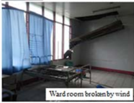
Ward room broken by wind
