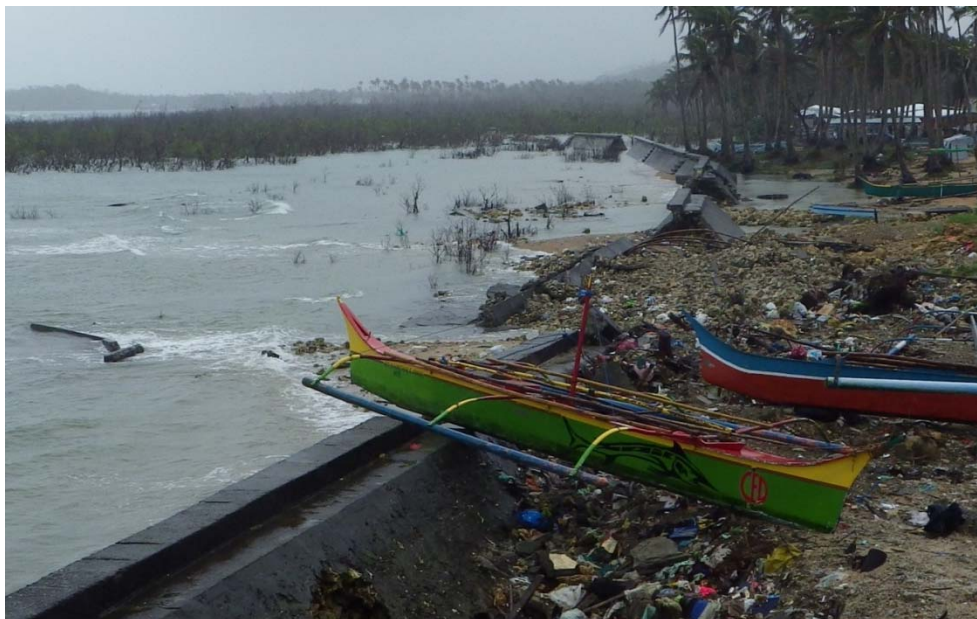
Fig.5-32. Damage to the Hernani seawall. Crest height 3 m above Mean Sea Level.
