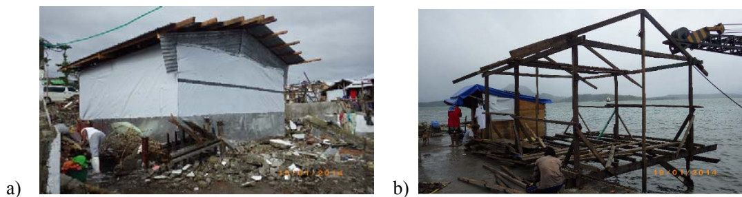
Fig.5-11. a) A house rebuilt with corrugated galvanized iron sheet and wooden studs, b) A house being rebuilt with debris.
