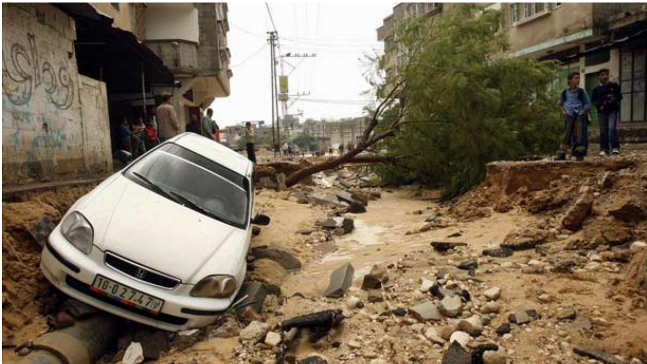
Figure 2.4: The disruptive and destructive impacts of a flash flood in the Gaza Strip, following 36-hours of heavy precipitation on 27-29 October 2008 (Source: UNDP/PAPP).
