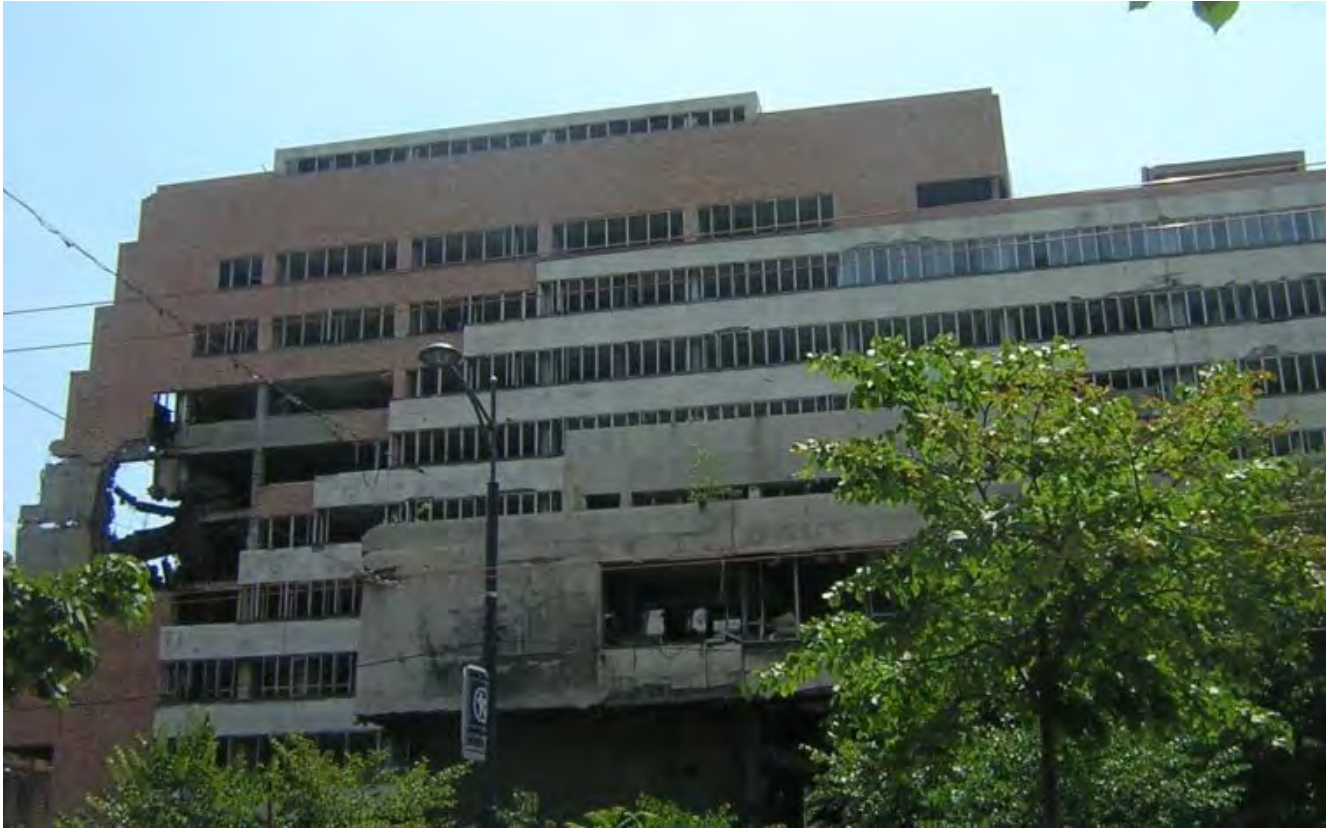
The General Staff building in Belgrade was bombed by Nato in 1999, and is now derelict. / bne IntelliNews
