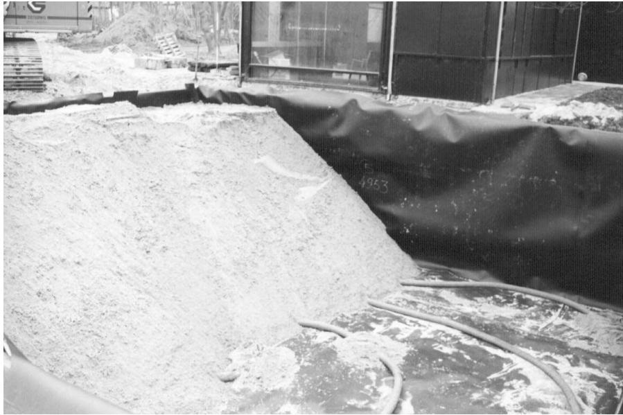
Figure 7.1: The construction of the testing site, where the drainage pipe is visible on the bottom of the testing site.
