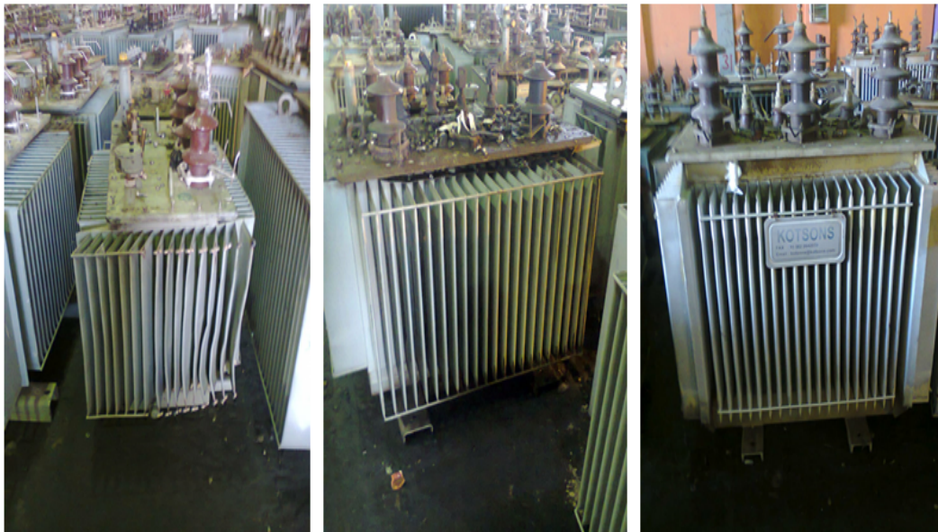
Fig. 9: Faulty DT samples from Baghdad electrical grid maintenance site as follows: pivot damage, oil leaks, and shorted winding.
