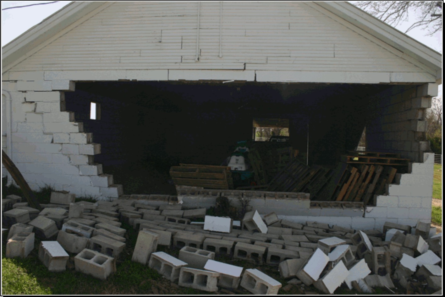
A concrete wall of a barn was blown in, a half mile south of Highway 9 on Western Avenue. Photo courtesy of Doug Speheger.
