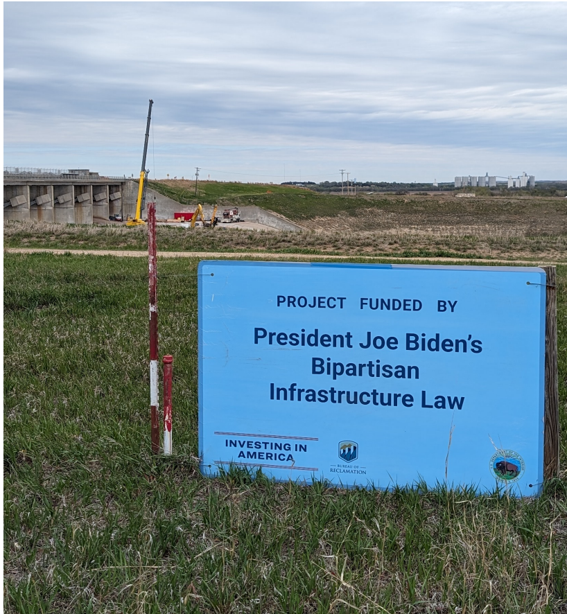
2024: Glen Elder Dam Spillway Extraordinary Maintenance Project, Pick-Sloan Missouri Basin Project, Kansas. BIL allocation of $14 million from BIL Aging Infrastructure/Extraordinary Maintenance.
