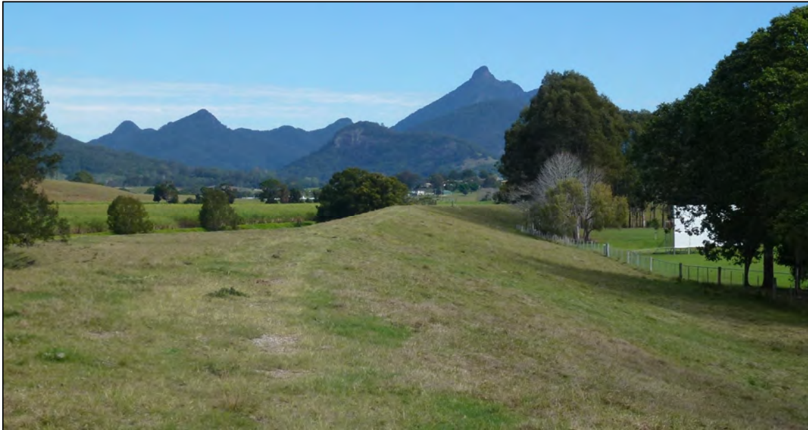
Plate 1 View looking west from Commercial Road showing earthen embankment section of Commercial Road levee
