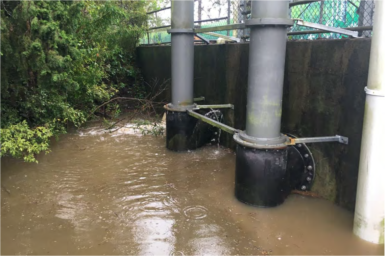
Lavender Creek Pump Station (3:00pm on 31 March 2017)
