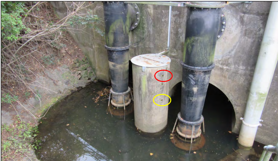
Plate 5 Lavender Creek Flood Pump Station 1 showing vertical intake structures (black vertical structures) and water level sensor (concrete chamber between the black intakes)
