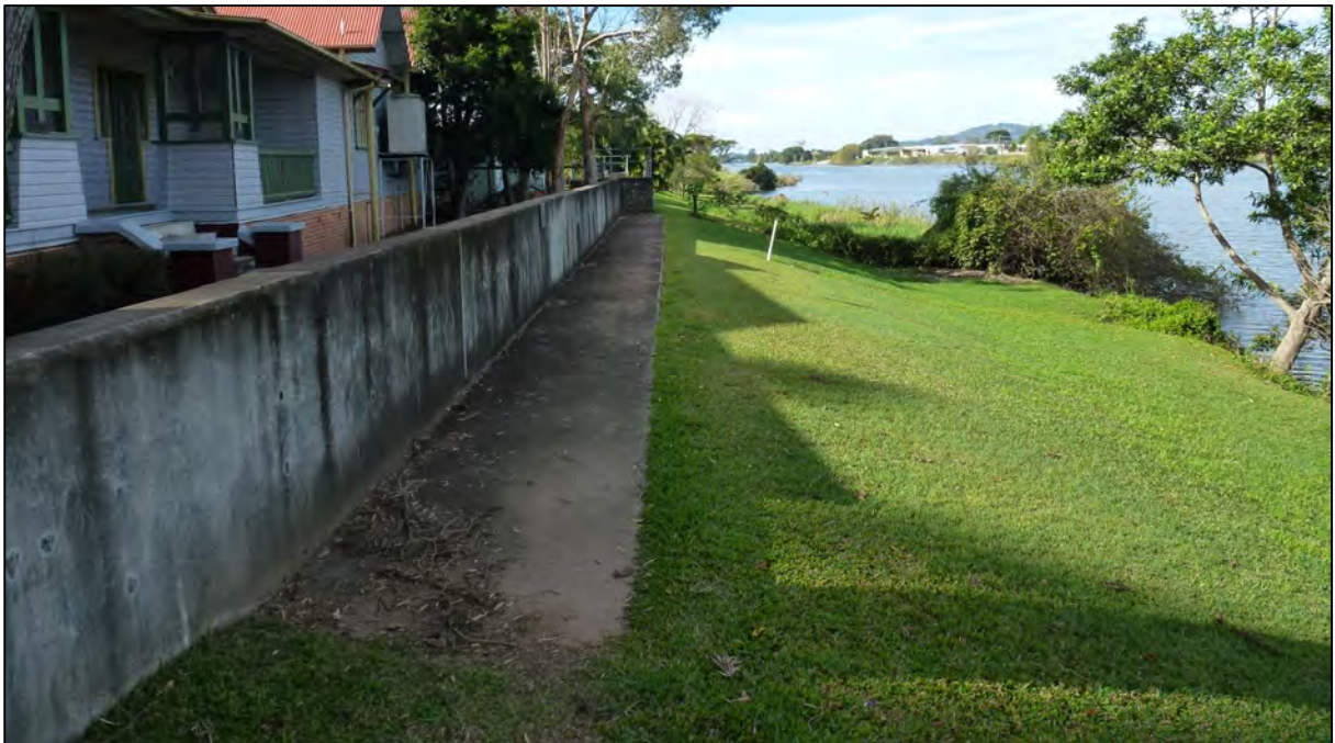
Plate 3 View looking north-east along concrete wall section of the East Murwillumbah levee
