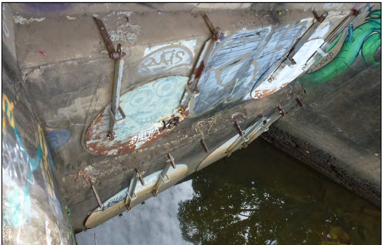
Plate 4 View showing flood gates on Tweed River side of Commercial Road culverts. The gates prevent water from the Tweed River “backing up” the culverts and inundating areas behind the levee
