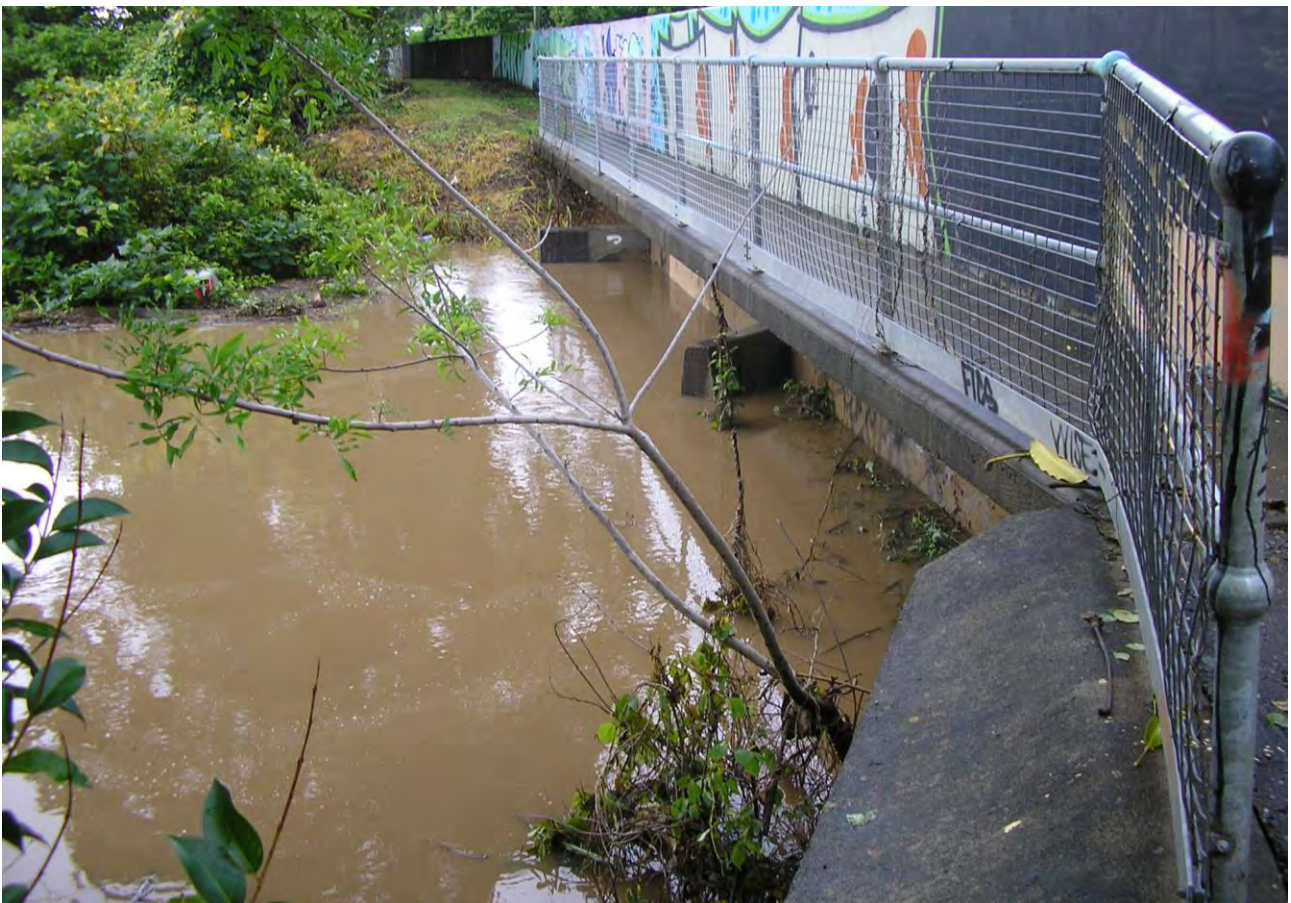
Elevated Tweed River Level at Lavender Creek outlet
