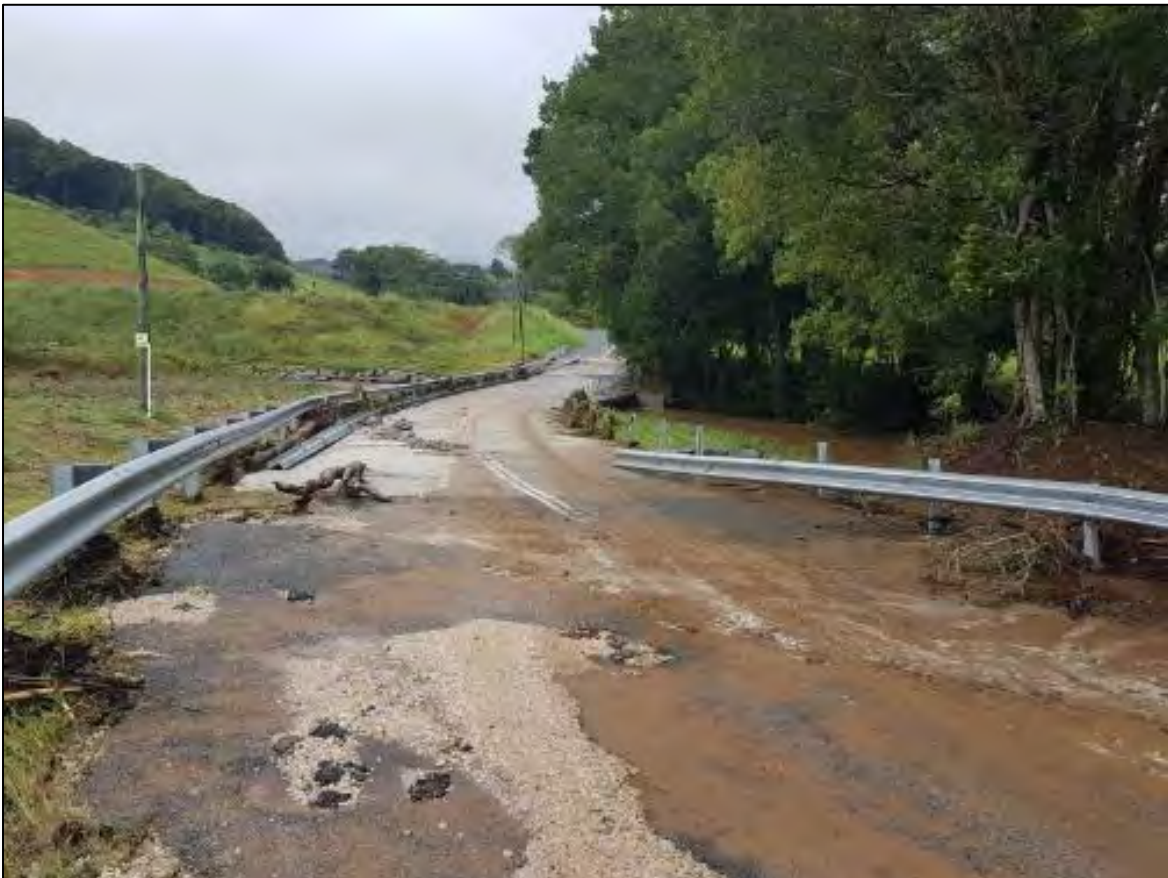
Photo 8: 01/03/2022 Cobaki Road Bridge damaged by the floods
