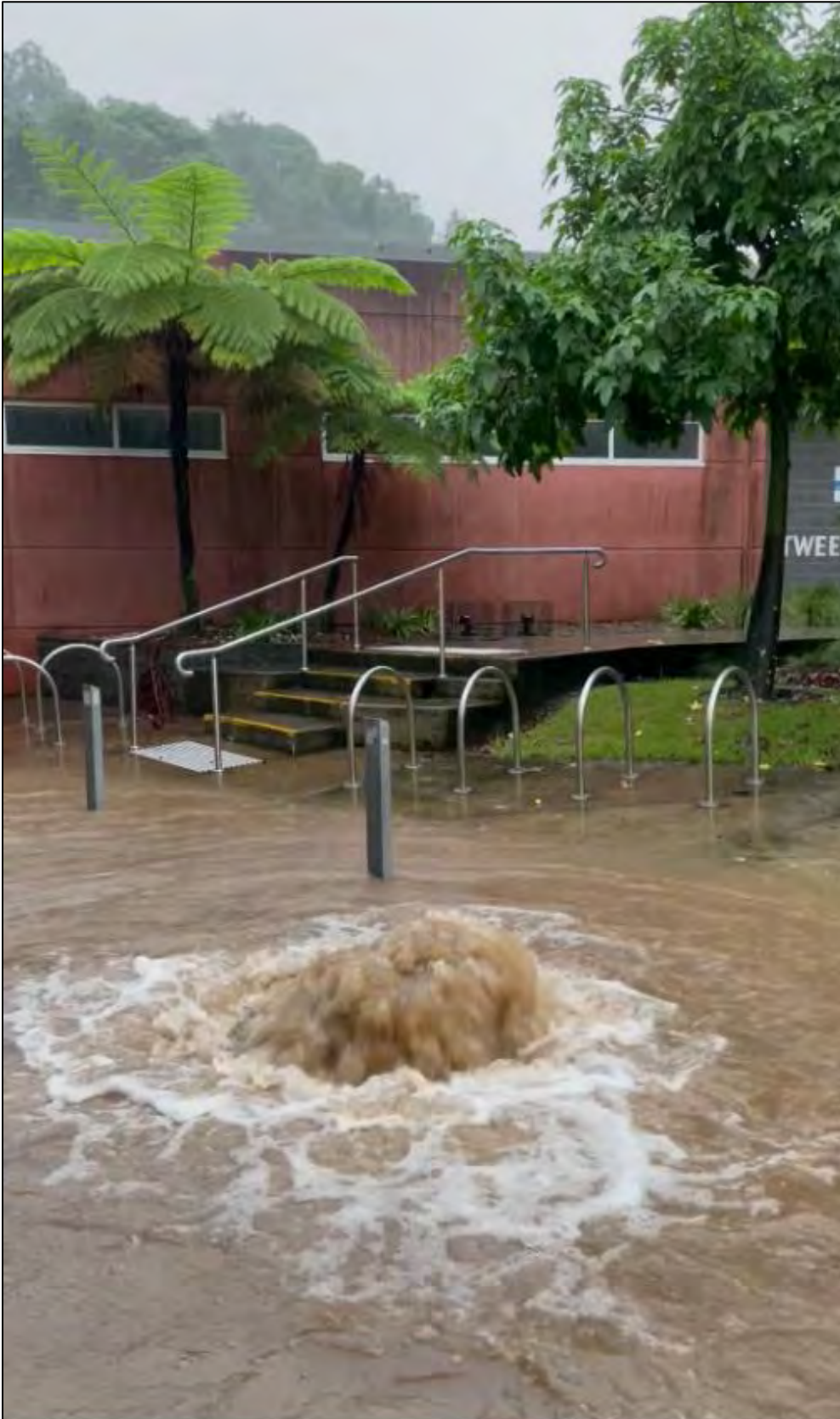
Photo 1: 28/02/2022 at 8:17 Pit surcharging at the Tweed Regional Aquatic Center
