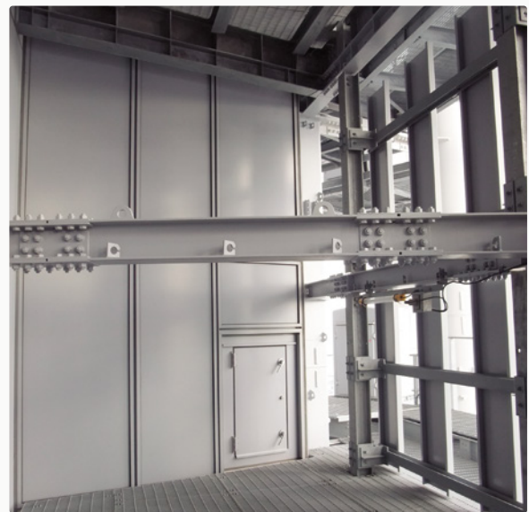
屋外機器置場(一例) An outdoor equipment site
