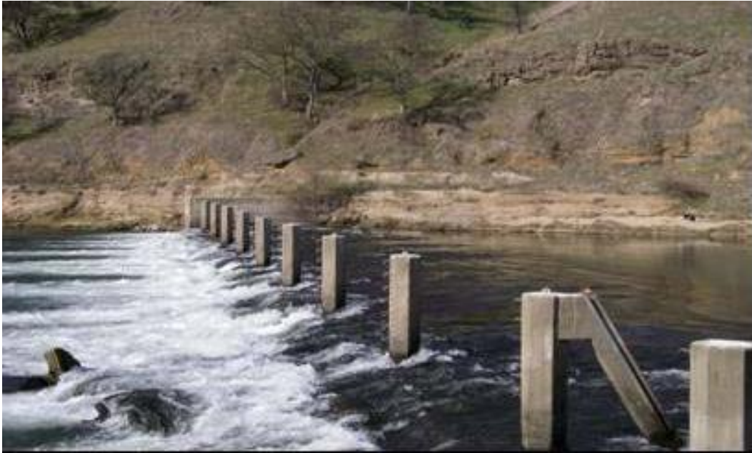
Figure 4-3. Concrete supporting piers in the river facing north on the left bank.
