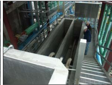
Unused Holding Tank
