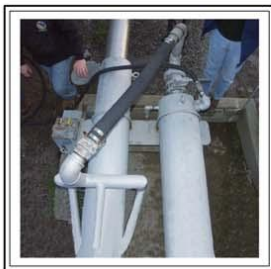
FLUSHING FLOW IS ADDED TO RELEASE PIPE - TYPICAL OF SWP AND CVP RELEASE SITES
