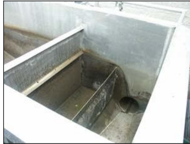
Sample Tank Drain
