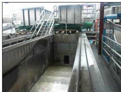
Holding Tank Drain
