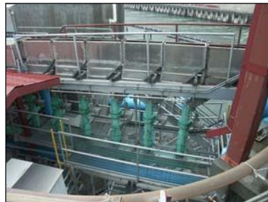
Flume Dewatering Valves
