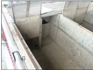
Raceway Water Level Control
