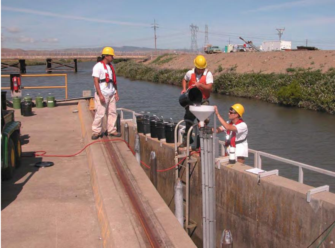
FIGURE 4.—Reclamation fishery biologists transferring Chinook salmon into insertion tubes in front of bypass No. 4 at the Tracy Fish Collection Facility.
