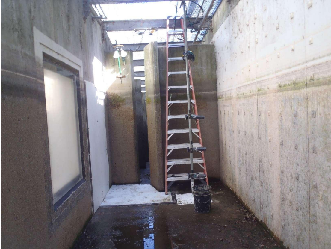
Appendix F Figure F24. The video station in the north ACID fish ladder for monitoring winter-run passage in 2016.
