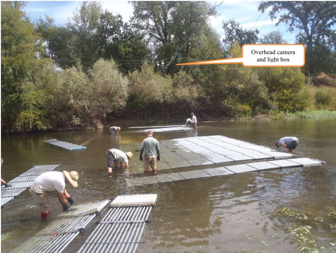
Appendix F Figure F5. The Cow Creek video station new resistance board weir under construction in fall of 2016. Note the height of the overhead camera and lights, destroyed by flooding later in season.
