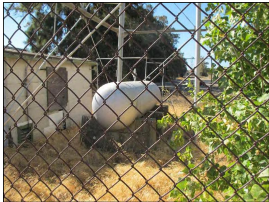
Photo 7. View of one propane tank west of the pump house facing south. Tank holds approximately 1,000 gallons.
