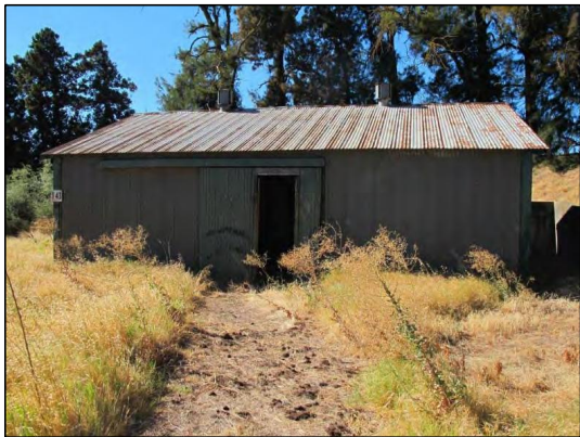
Photo 3. Exterior of the former flammable materials storage building facing south. No hazardous materials or waste was observed.
