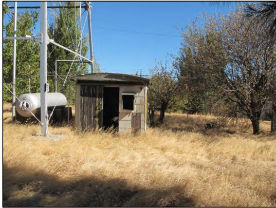
Photo 5. View of exterior of the pump house near the water tower in the central portion of the site facing north. Pump house contained one groundwater supply well, dismantled well pump, and associated plumbing, and one air compressor.
