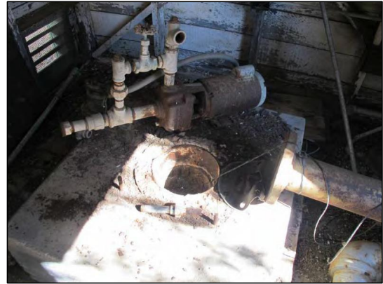
Photo 6. One 8-inch groundwater supply well with dismantled pump in the pump house. No well lid to protect groundwater was observed and groundwater level was estimated at approximately 8 feet below ground surface.
