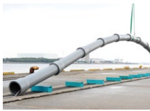
Installed earthquake-resistant ductile iron pipes for the first time in the U.S.
