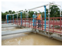
Constructed water treatment facilities in Myanmar
