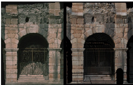
fig. 8 Comparison between the two ortofoto: on the left ortofoto from photogrammetry and to right ortofoto from laser scanner
