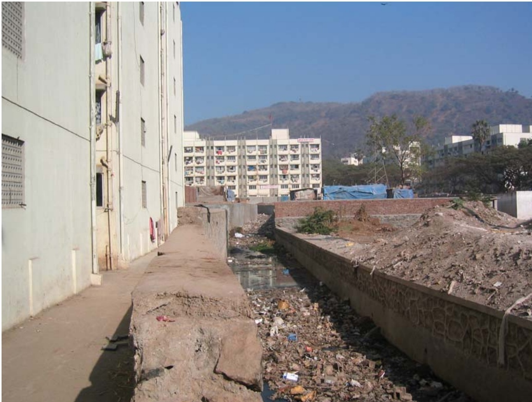
Environmental problems at resettlement site
