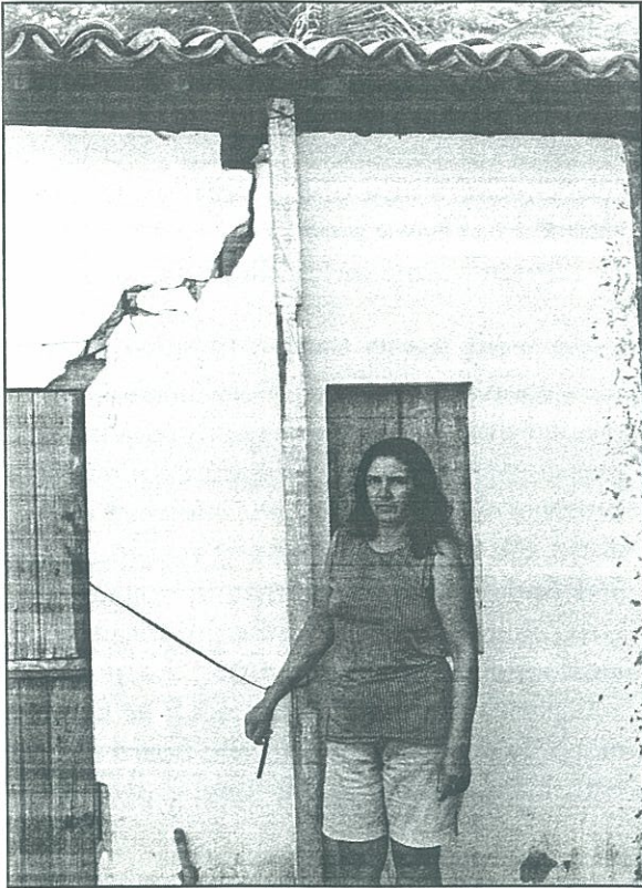
A resettler showing the cracks in her house
