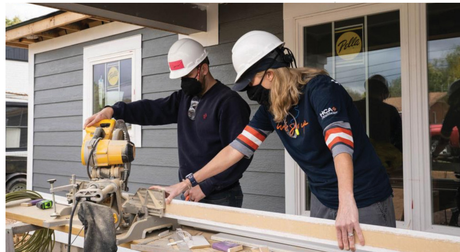
Above: Twenty-six HCA Healthcare volunteers, including Spencer Jones and Bev Sears (pictured), spent a day building a Habitat for Humanity home in Columbia, Tennessee.
