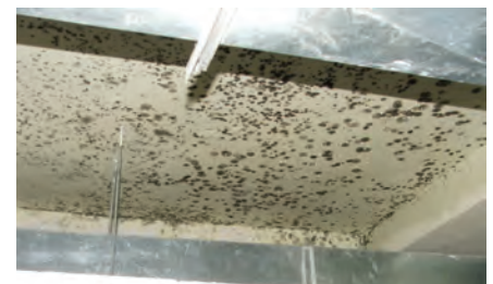
Mold growth in bathroom at Afghan Air Force University, March 2015. (SIGAR photo by Javed Khairandish)
