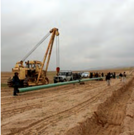
The Mazar-Sheberghahn pipeline was rehabilitated with the assistance of TFBSO. (GIROA photo)
