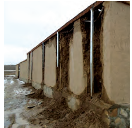
Defective materials and construction methods , as well as poor planning and oversight, were responsible for the exterior deterioration of the dry-fire range, which was caused by water penetration and required that the facilities be rebuilt. (NPTC photo)
