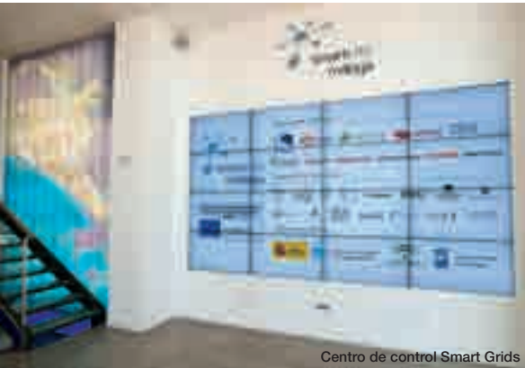
Centro de control Smart Grids
