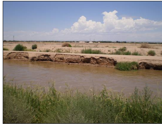
Photograph 3-3. Canal Bank Erosion and Caving.
