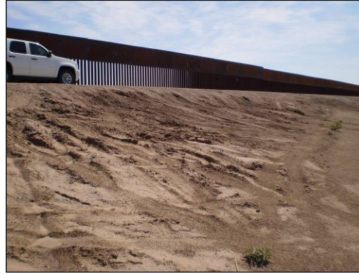
Photograph 3-12. Rutted Levee and Vega at the West End of Segment K-5.
