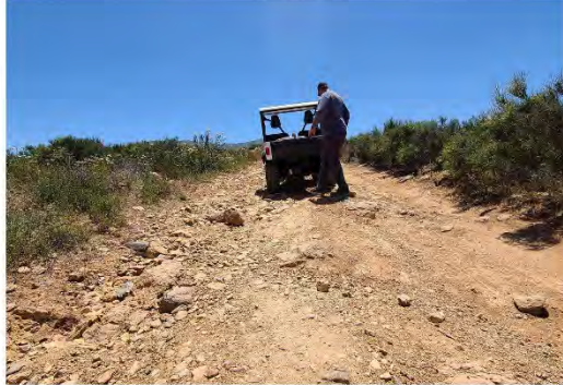
Water Cutout (WC6)
