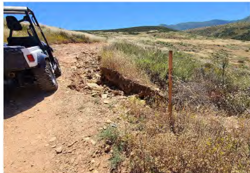
Water Cutout 1 (WC1)
