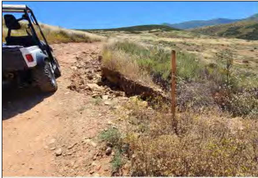
Photograph 2-2. Example Water Cutout Location
