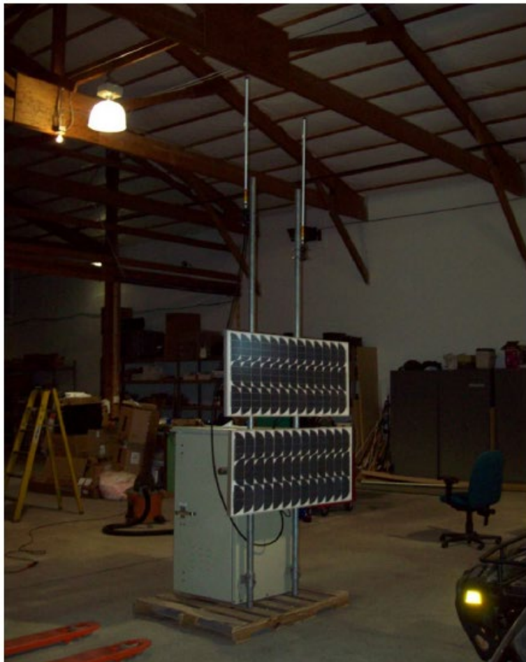
Enclosure 1: Representative Photograph of TCNS Shelter
