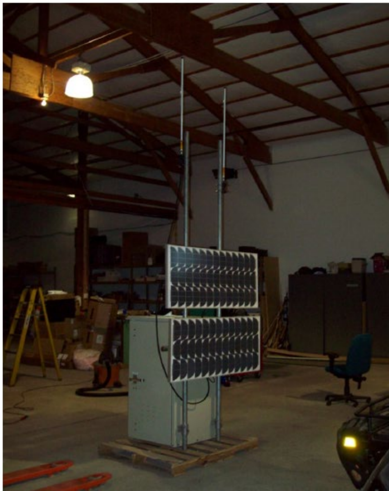
Enclosure 1: Representative Photograph of TCNS Shelter
