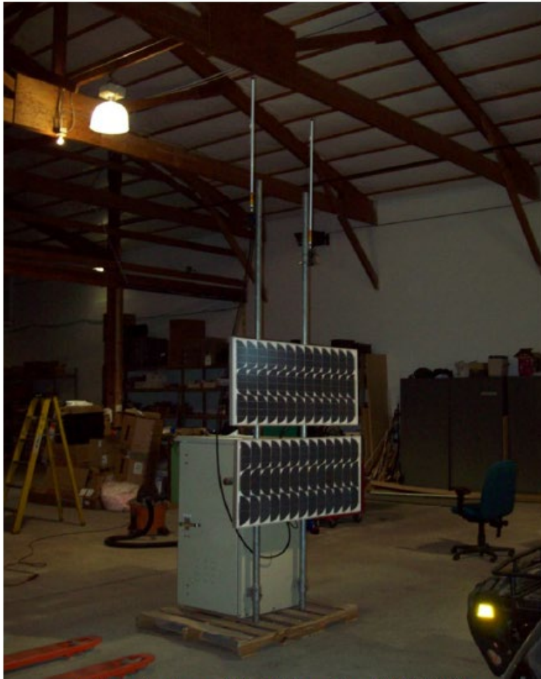
Enclosure 1: Representative Photograph of TCNS Shelter
