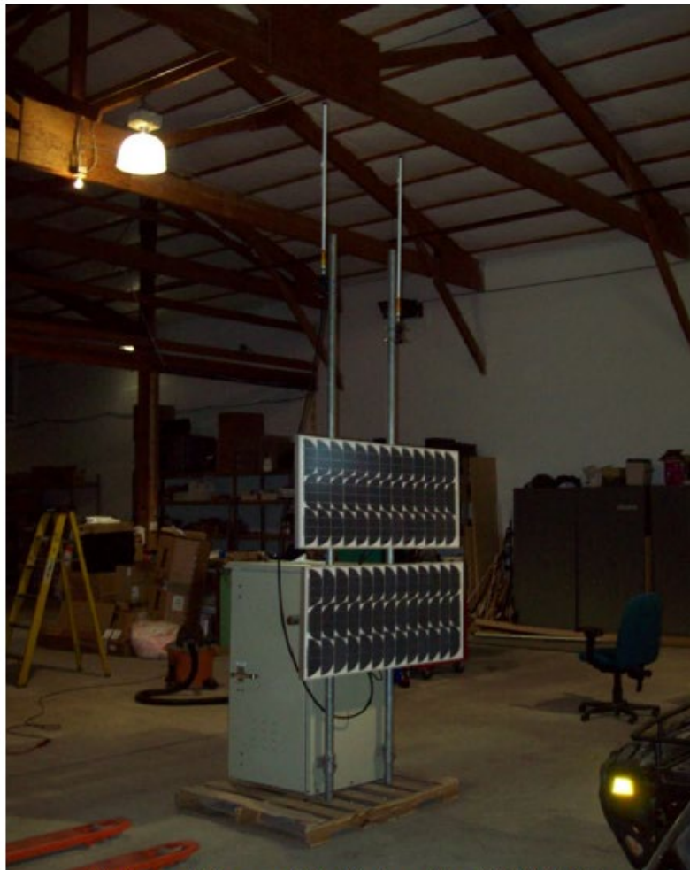
Enclosure 1: Representative Photograph of TCNS Shelter
