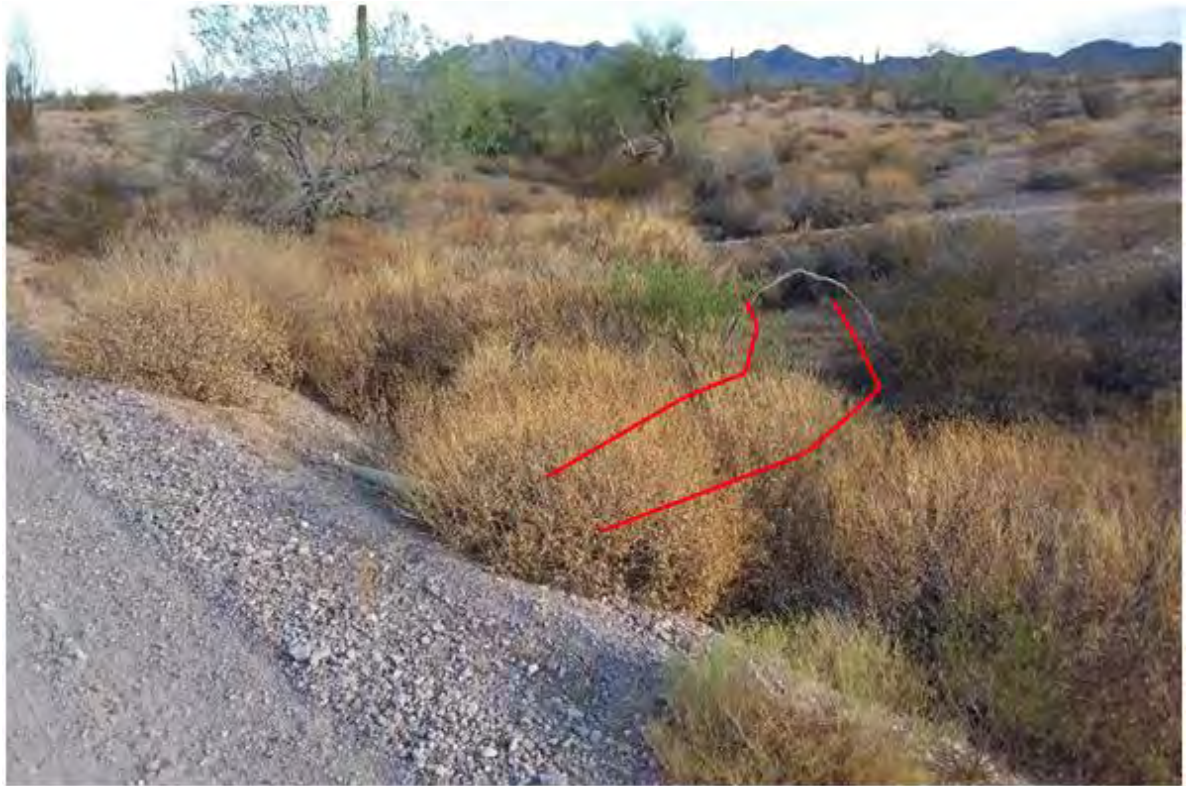
Figure 286. Photo point a23w1 looking upstream Channel flows into a culvert under road
