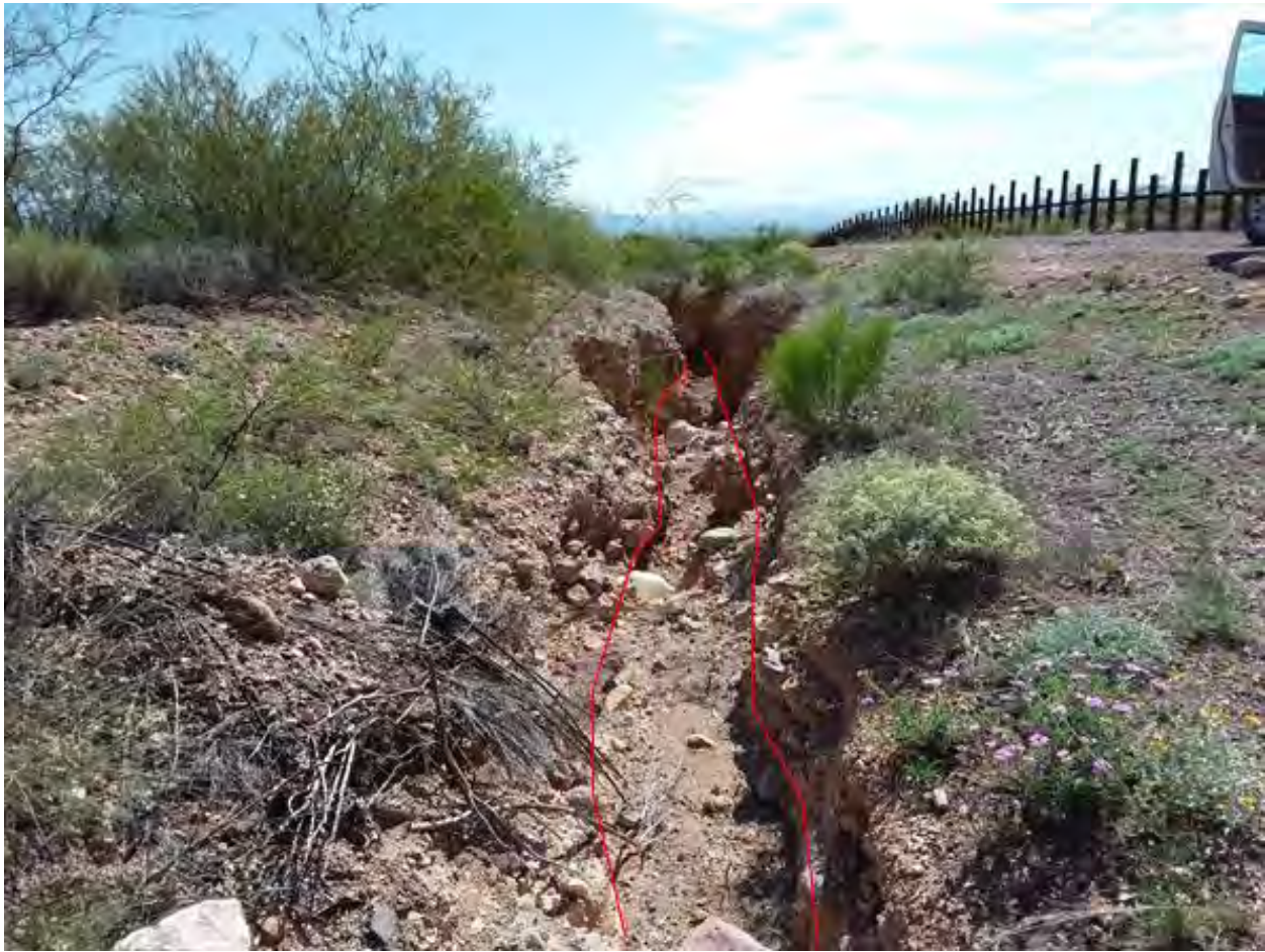
Figure 851. Photo point d2 at ditch forming along road
