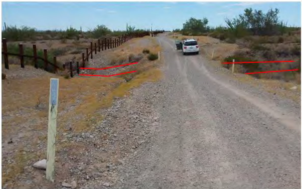
Figure 182. Photo point a14w1 looking west There is a double culvert under the road here
