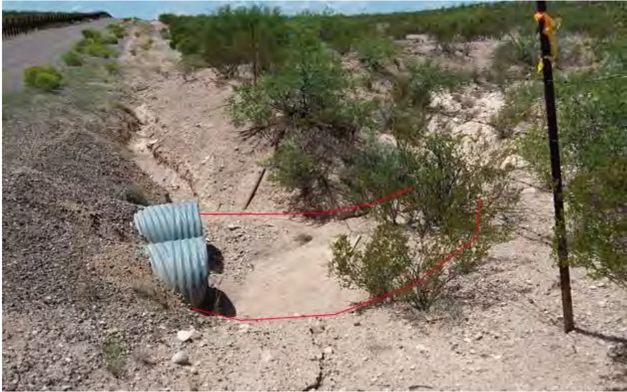
Figure 903. Photo point e8a looking west
