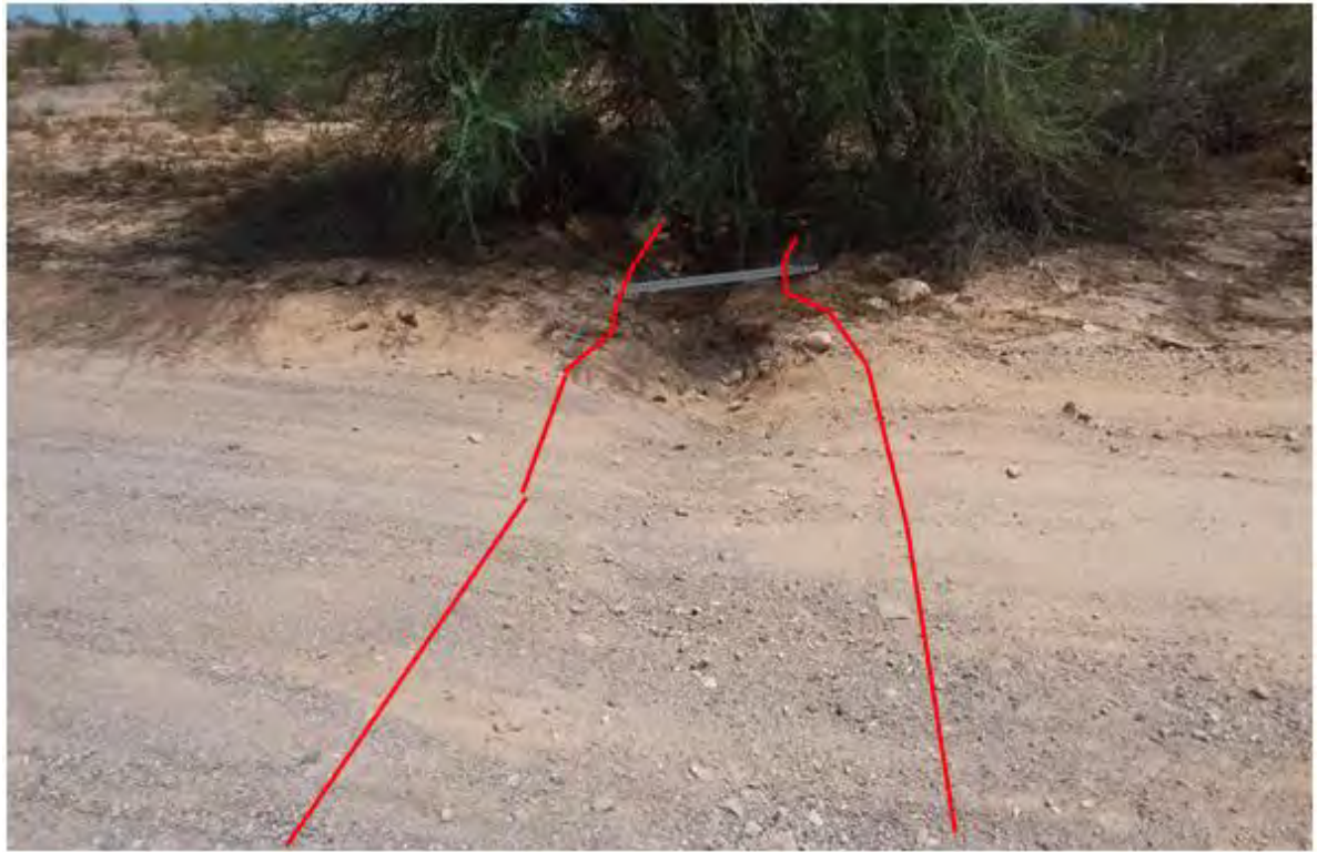
Figure 680. Photo point c3 looking upstream This only shows one of the trib
