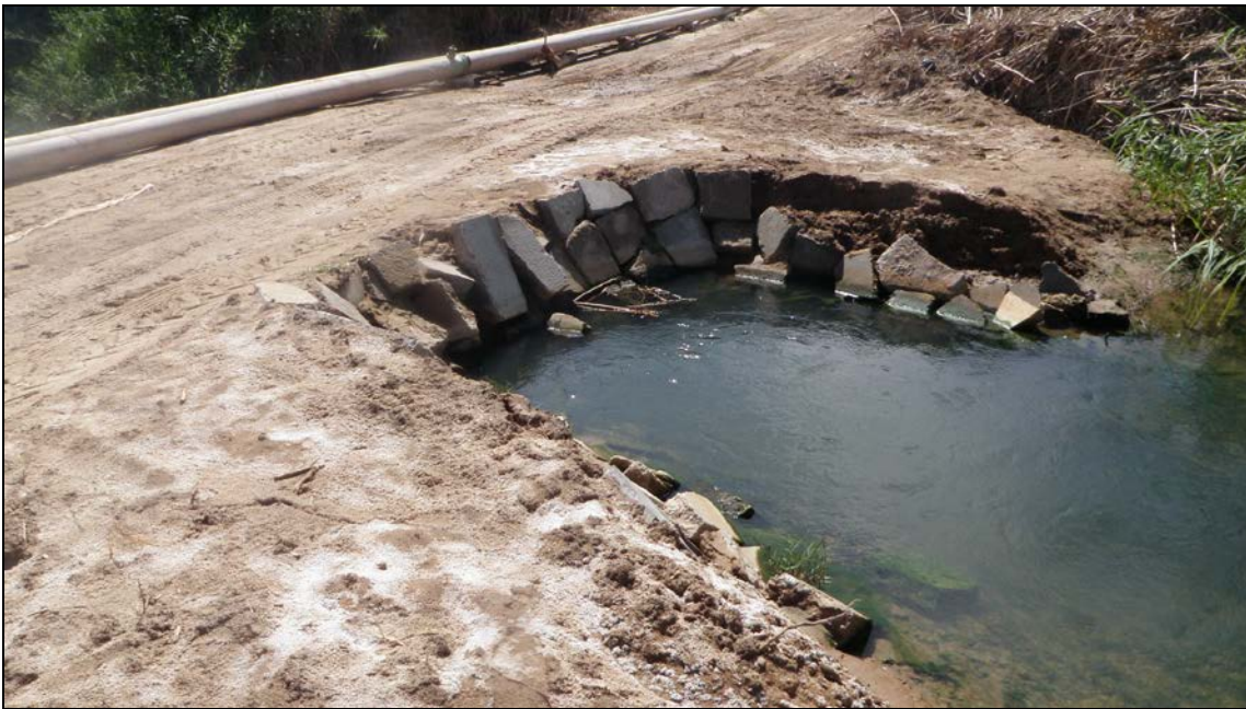
PHOTOGRAPH 9: Detail of a makeshift culvert crossing jurisdictional wetlands in central grubbed area.
