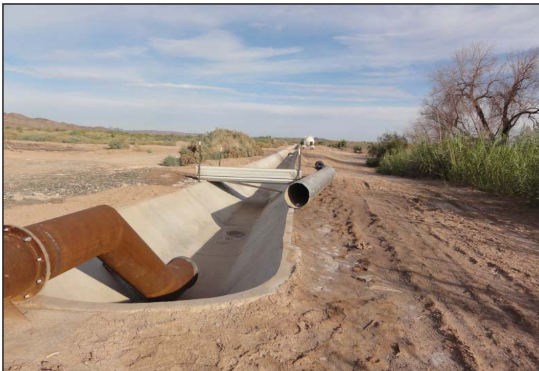
PHOTOGRAPH 2 Pumping Station Outlet Flows into eExisting Irrigation Channel
