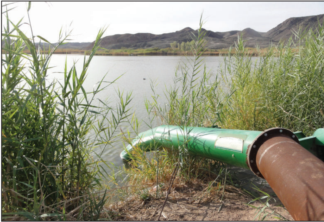
PHOTOGRAPH 5 Mittry Lake: Irrigation Pump
