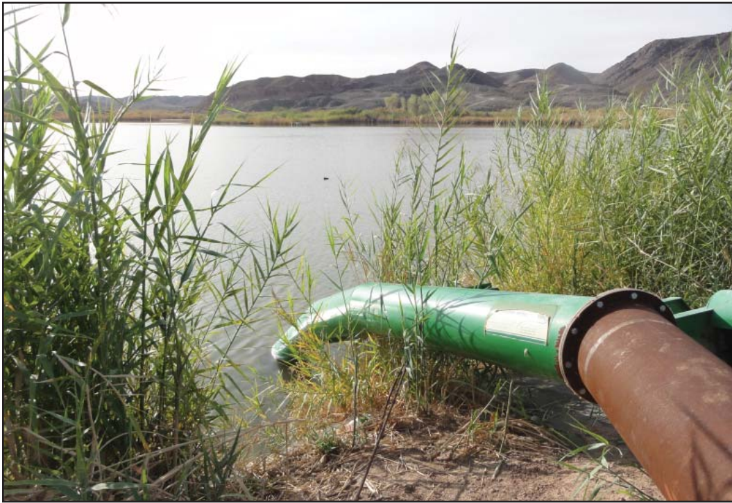
PHOTOGRAPH 1 Pumping Station Inlet at Mittry Lake
