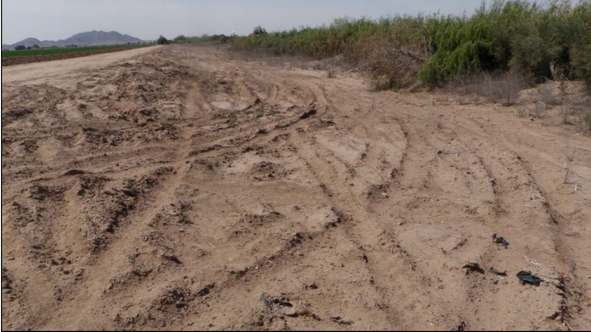
PHOTOGRAPH 4: Grubbed area adjacent to access road in southwestern corner of the project area.
