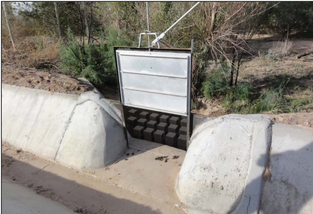
PHOTOGRAPH 4 Manually Operated Diversion Outlet
