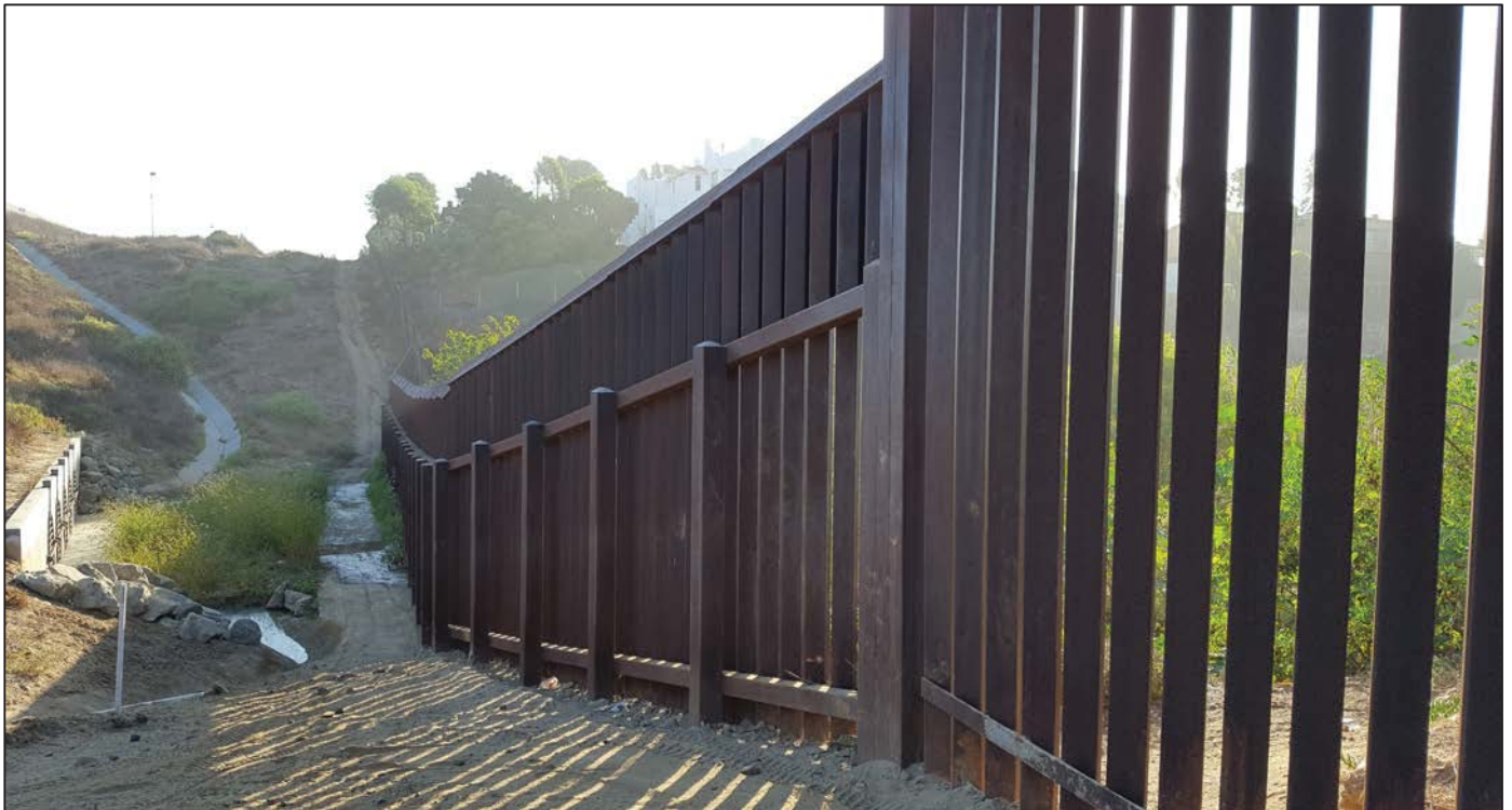
Photograph 2.4 Proposed Primary Fence Types. Additional example of bollard style fence installed at west end of Study Area.
