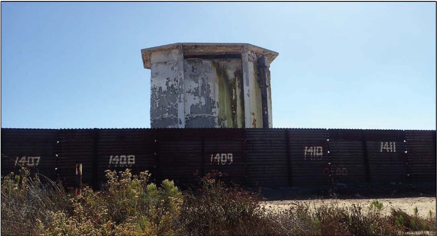
Photograph 2.1 Existing Primary Fence. View of the landing mat style fence planned for removal.
