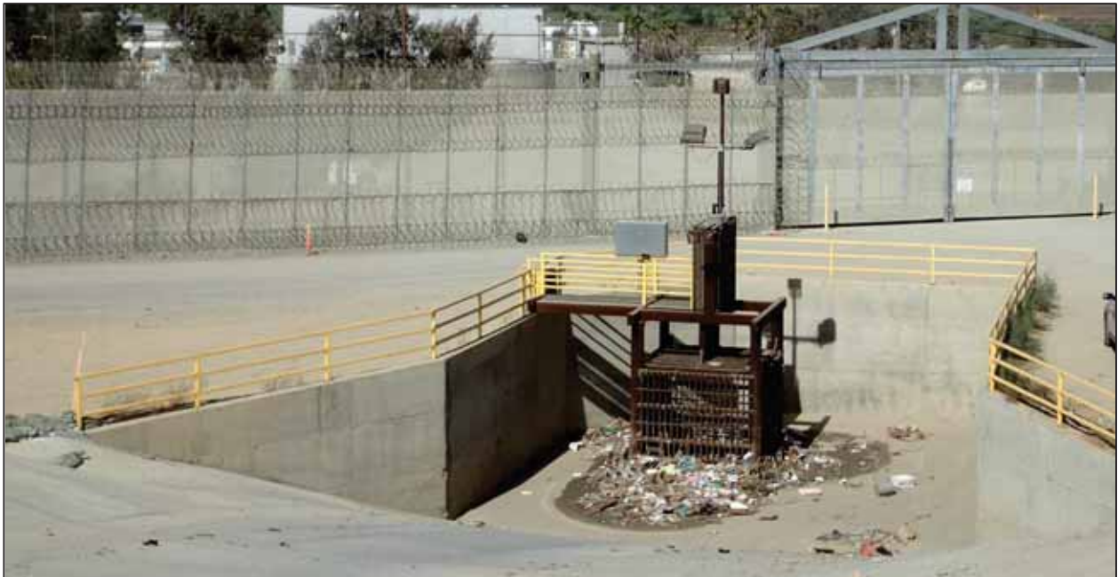
Photograph 16. Non-jurisdictional concrete drainage, located to the southwest of the waste treatment facility. View facing north. Photograph taken on October 10, 2017.
