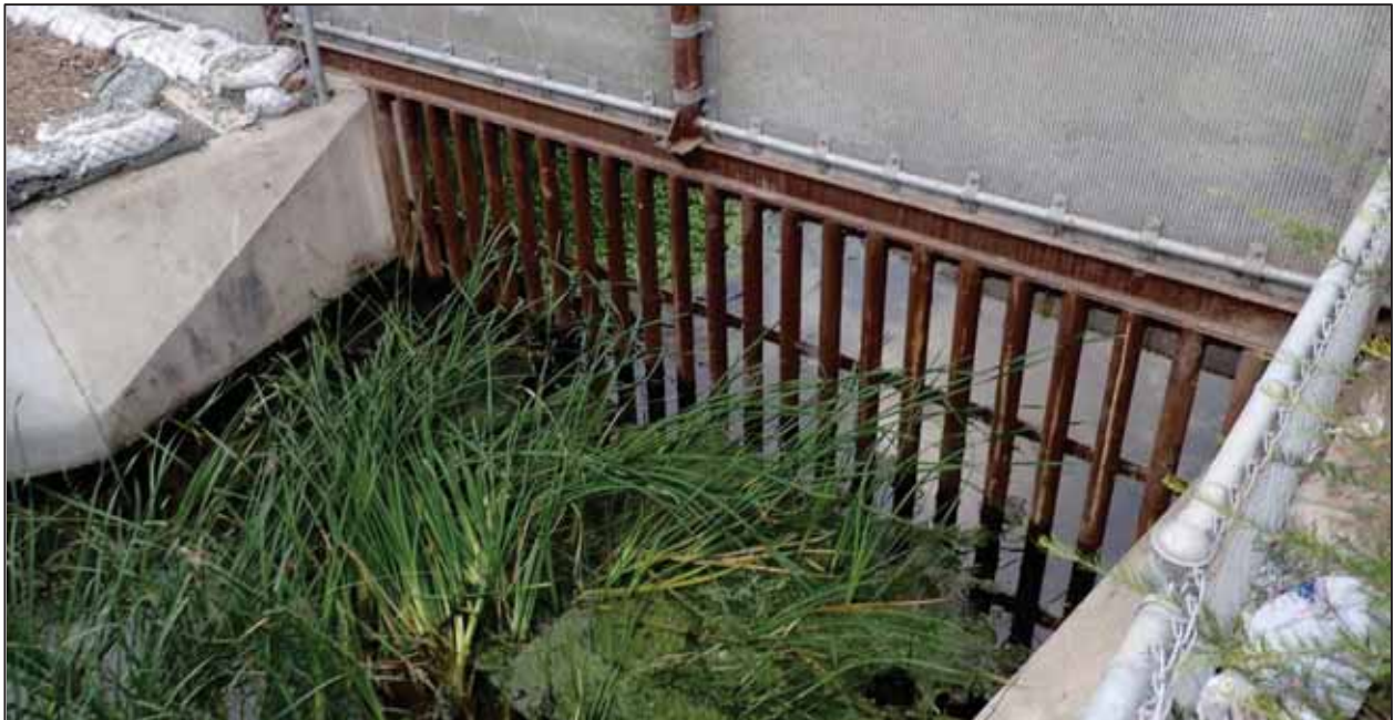
Photograph 6. Image is of wetland ditch W03, located in a concrete drainage channel near the north bank of the Tijuana River, approximately 0.4 mile west of the San Ysidro POE. Sufficient sediment has accumulated to support vegetation dominated by cattails and dock. Based on aerial imagery, it is expected that W04, the eastern portion of the concrete channel, is similar in hydrology and vegetation to W03. View facing south. Photograph taken on October 12, 2017.
