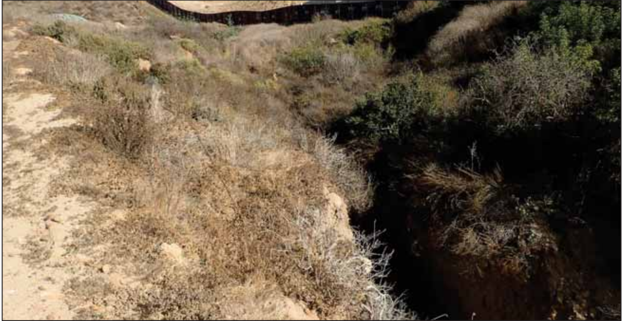
Photograph 7. Image depicts the narrow, deeply incised upper reach of S01, approximately 0.75 miles east of Friendship Park. View facing south. Photograph taken October 9, 2017.
