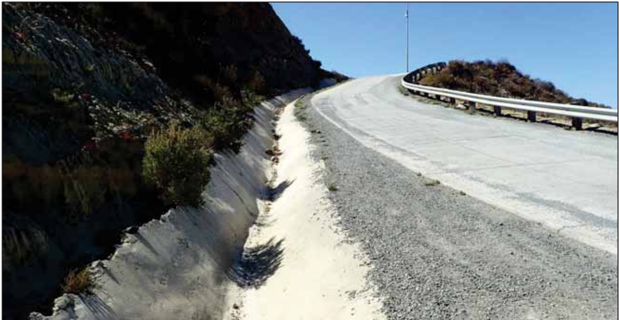
Photograph 14. Image depicts an example of a concrete, V-shaped drainage on the eastern slope of Bunker Hill. Such features are constructed in uplands and drain roadsides and other uplands. Such features were considered non-jurisdictional. View facing west. Photograph taken October 10, 2017.
