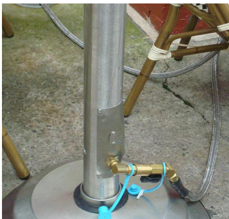
Flexible gas hose connector at portable gas heater (seen without protective cover)
