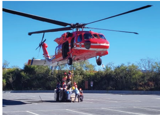
Sling loading of building materials for supporting the construction of mountain cabins by the CPA
